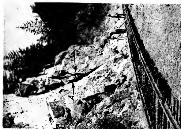
(c) Preparing to trim an unstable rock block (A) which contains sufficient volume to cover the track. With the steeply dipping joint potential failure is obvious.
