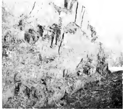
(d) Bedded rock dipping into slope. Ravelling will occur due to cantilever type toppling failure. Slope angle of 70^{\circ} - 75^{\circ} suggested.
