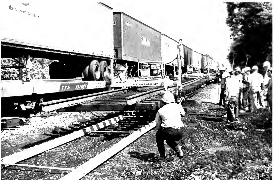
Upon completion of the grading, temporary track is again installed and the same track panel is returned.
