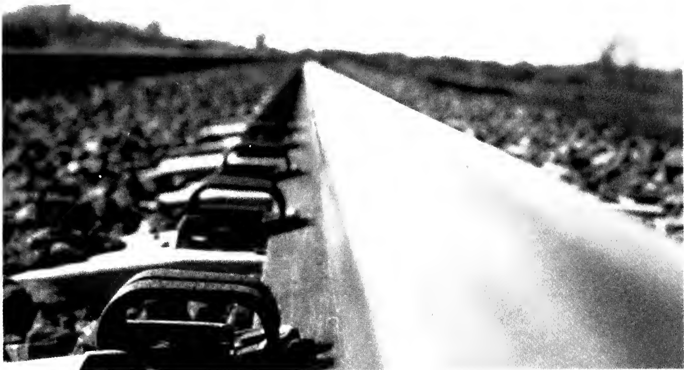
A section of the Hamersley Iron Railway between Dampier and Tom Price Mine, Western Australia
