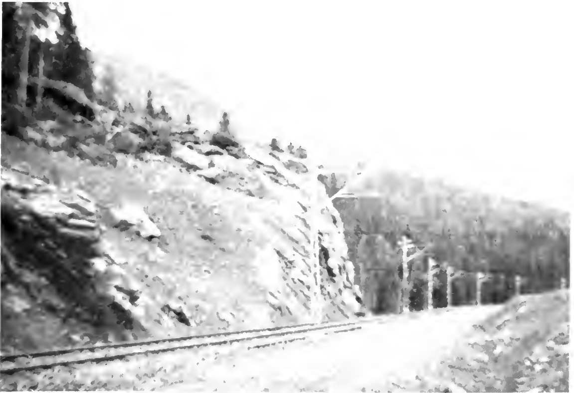
PHOTO. 7 View showing completed grade, track and overhead contact systems in vicinity of Km 97 (Wolverine River Valley).
