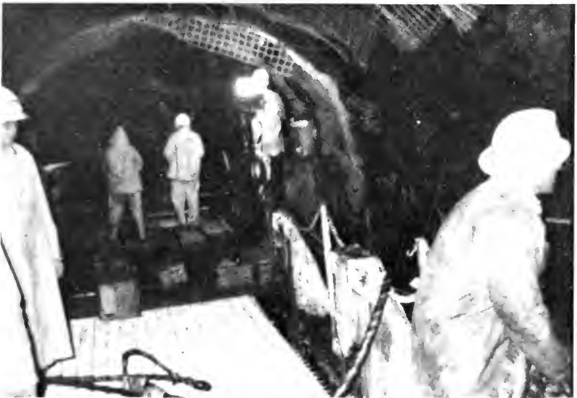
PHOTO. 8 View showing placement of wire mesh in the construction of the Table Tunnel.
