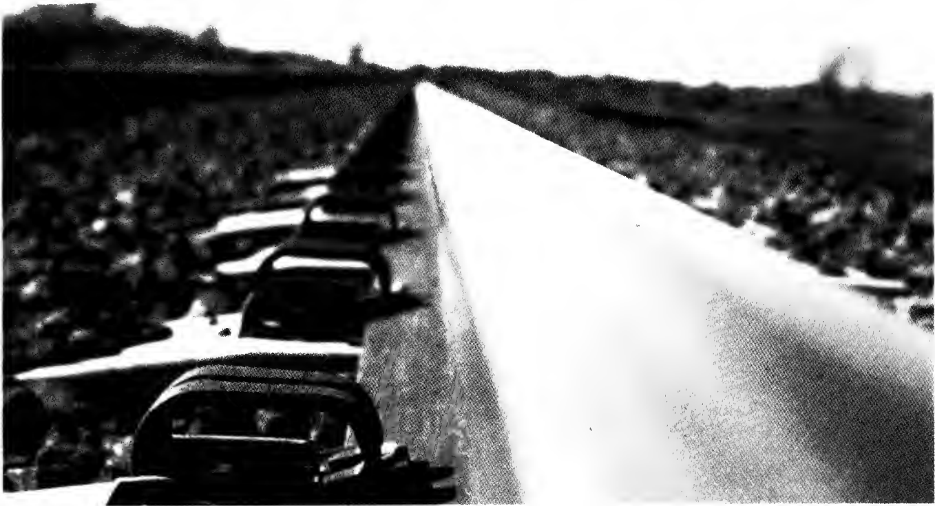
A section of the Hamersley Iron Railway between Dampier and Tom Price Mine, Western Australia
