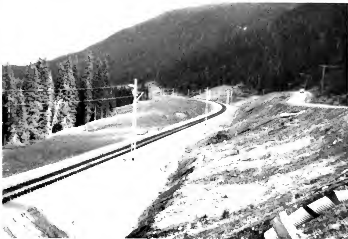
PHOTO. 2 View of completed track and overhead contact systems in the Table River Valley.
