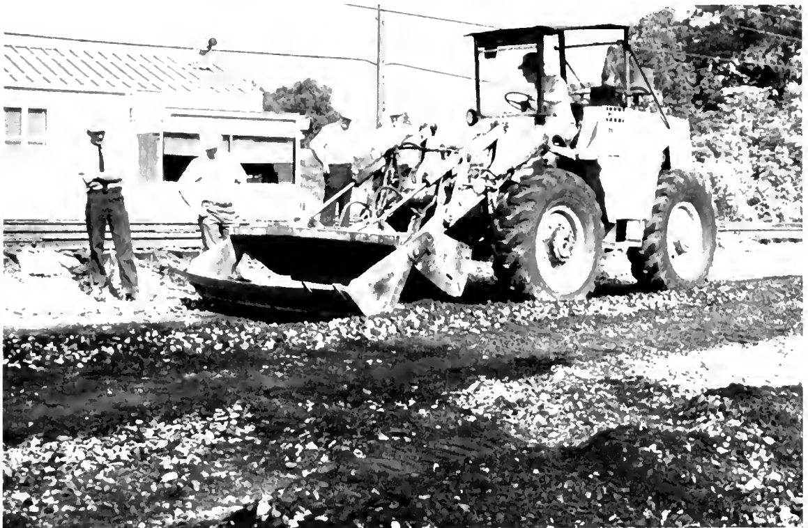
In addition to a tracked dozer, the Seaboard used a loader with a segmented bucket to assist in grading.
