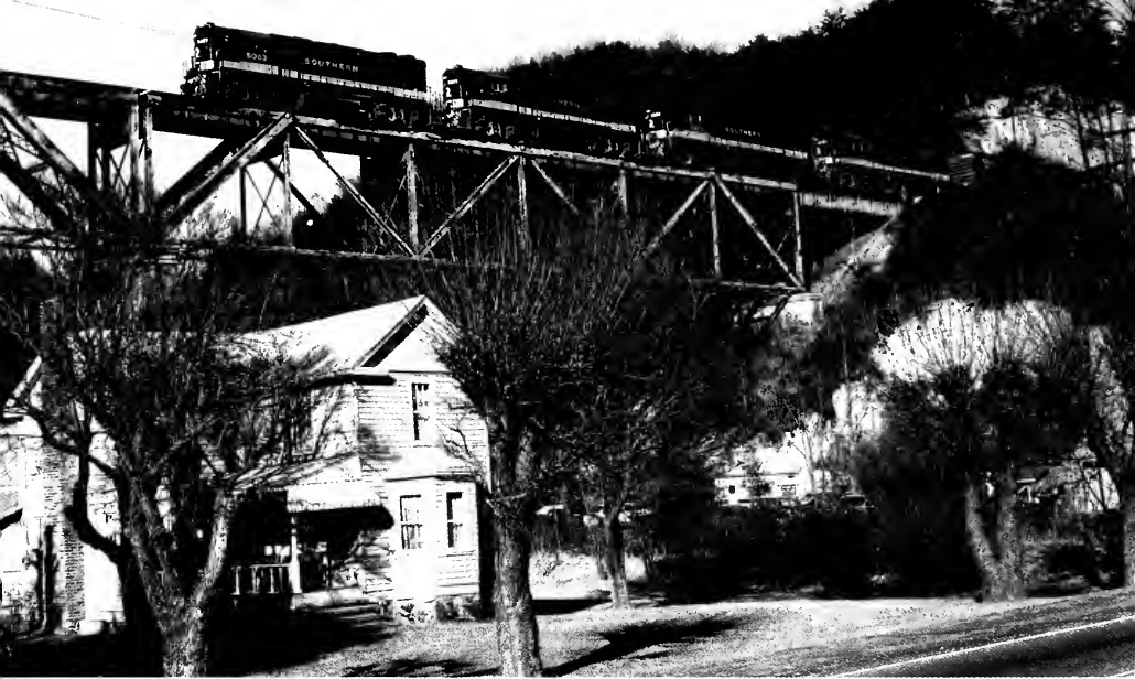
Figure 2 - Norfolk Southern freight heads for Canton, N.C. from Asheville over high deck truss bridge.
