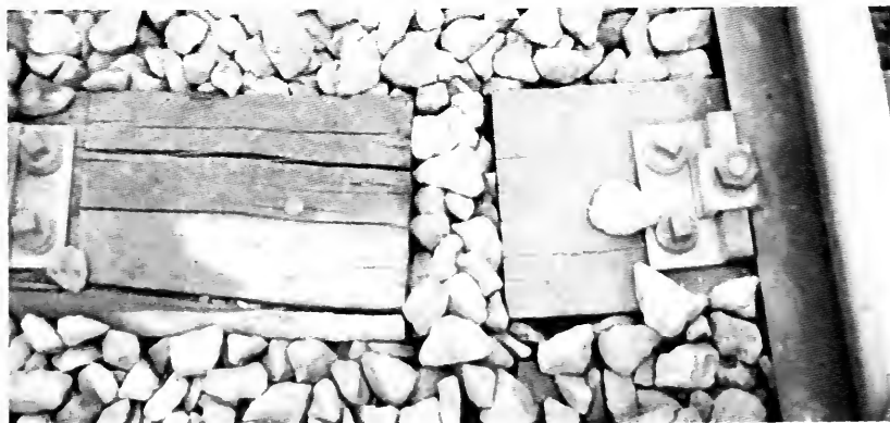
Oak tie (left) and Azobe tie (right), in France in 1957.
