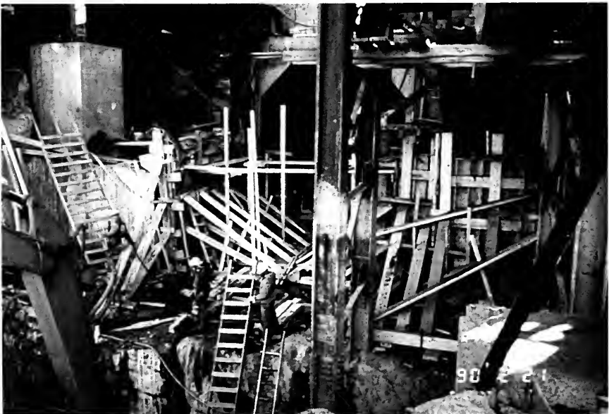
Photo 5. View of obstacles encountered at north tunnel access area.
