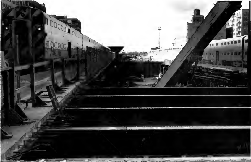
Photo 3. LaSalle Street Station, a three phase project which will completely renew the track, structure and train control system for the station.
