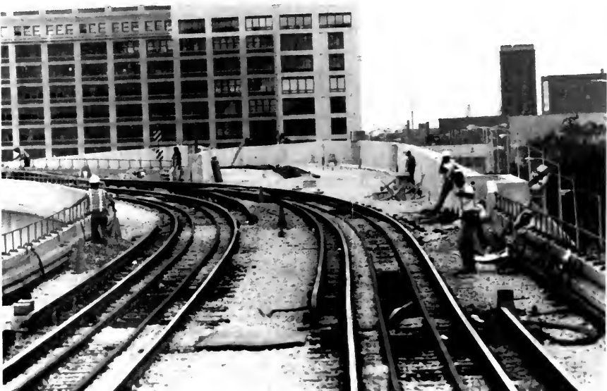
Photo 4. Work nearing completion on CTA's Southwest Rail Line which will service southwest Chicago including Midway Airport.
