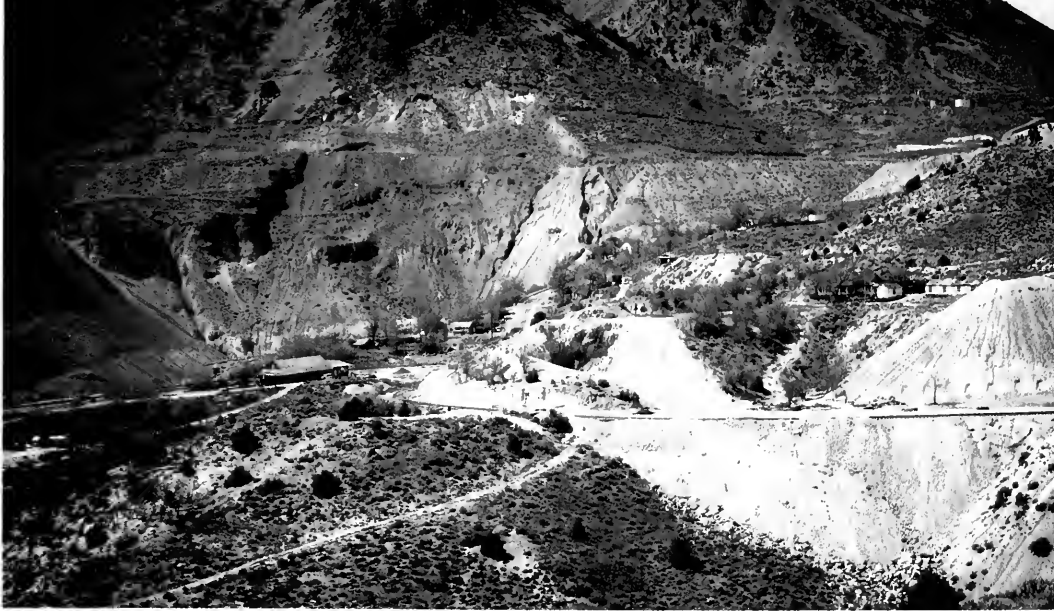
Photo 1: Overall view of by-pass project with Gold Hill Depot in background, at left.
