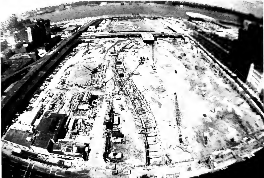
Photo 4. Aerial view of Long Island Rail Road west storage yard prior to its construction. Alignment of west side tunnel is visible.
