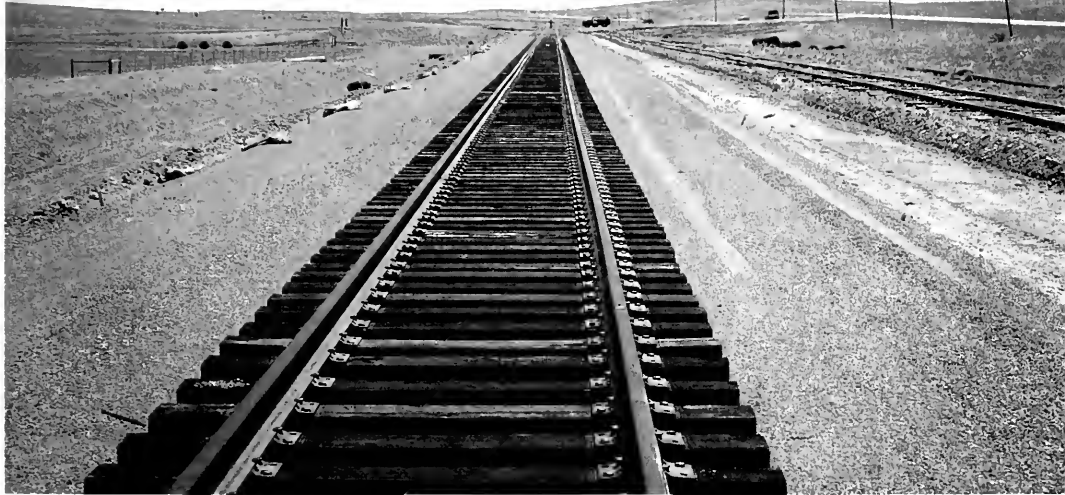
New wood tie track before ballasting on C&NW coal line west of Lusk, Nebraska in 1984. Old Chadron-Casper Line is on right.
