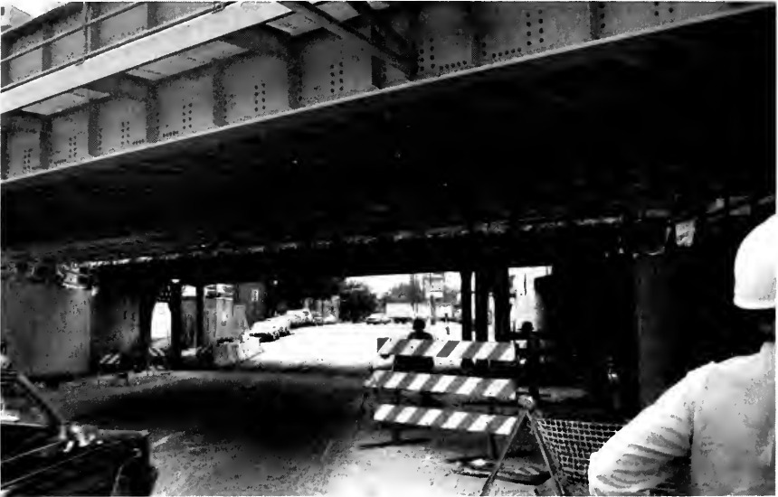
Photo 1. Metra Bridge Renewal in progress. More than 35 bridges slated for renewal on Metra's north and northwest lines.
