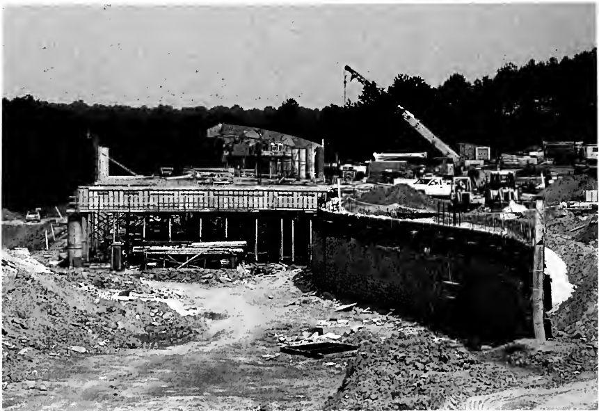
View of Indian Creek Station with glue laminated roof beams and sine wave wall in foreground.
