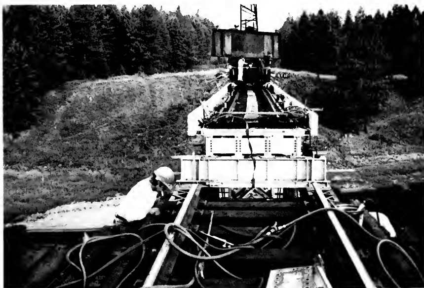
Figure 3. Progression of replacement from wood tie deck to concrete ballasted deck on Bridge 208.
