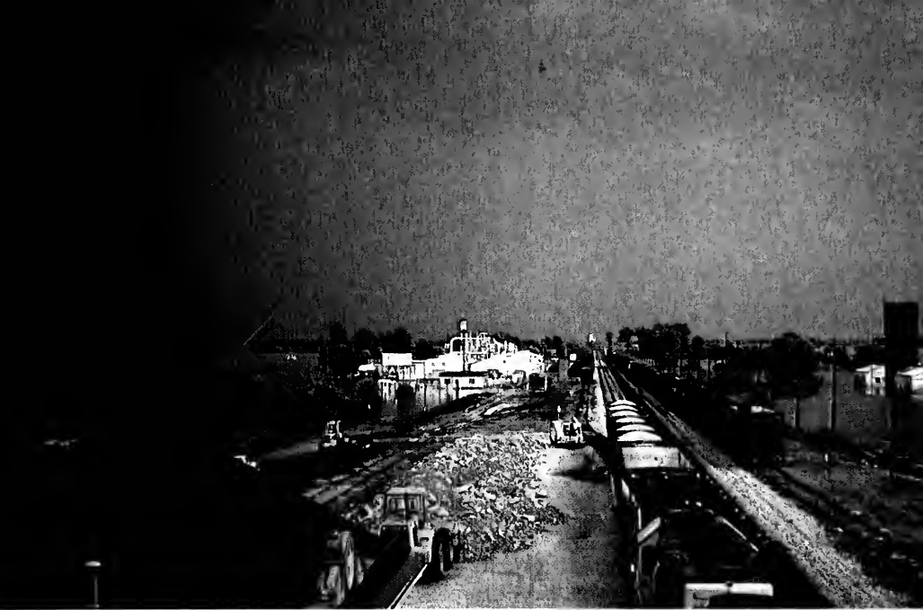
Rain clouds threaten further flooding as Santa Fe work train with Jordan spreader and ballast cars prepares to leave Henrietta, Missouri July 31, 1993.
