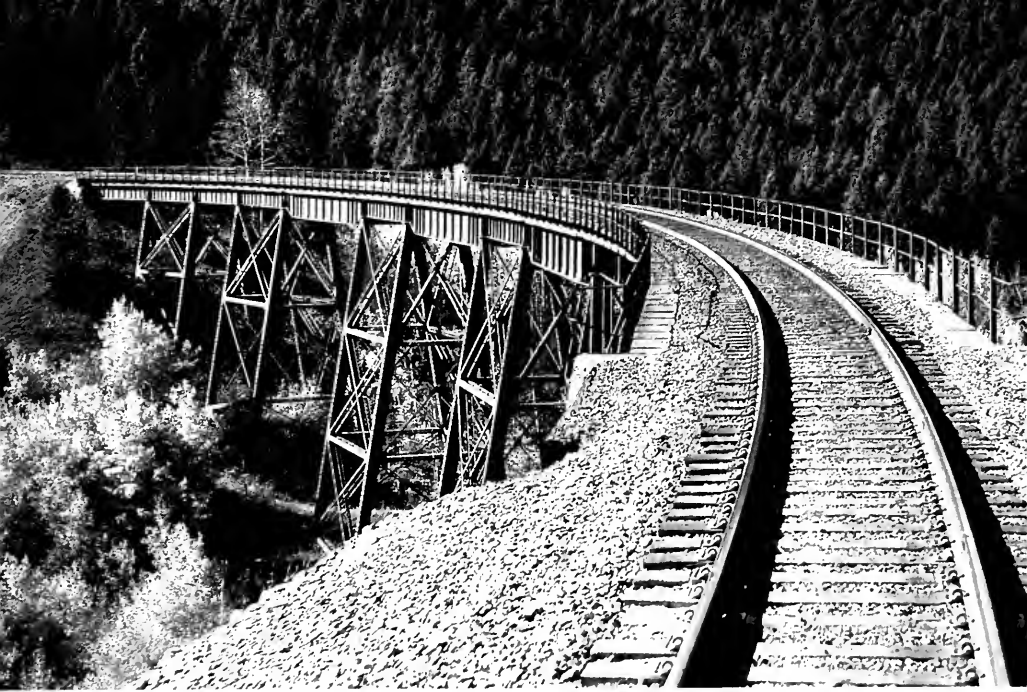
Photo 1: Large curved steel viaduct on upper portion of eastern approach to Mullan Pass on Montana Rail Link.
