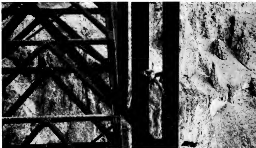
Figure 4. A Burgess & Niple bridge inspector descends fixed ropes to gain access to pin connections on the Perrine Bridge in Idaho.
