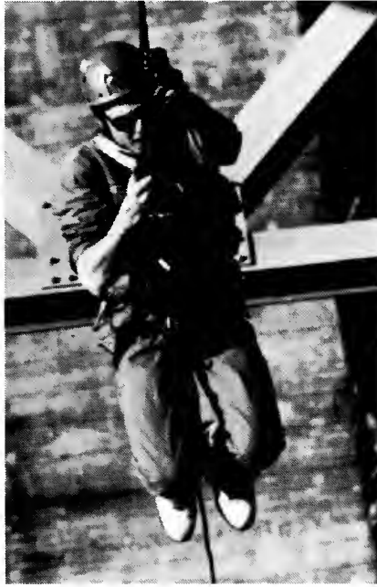
Figure 5. A CALTRANS engineer/technician uses mechanical ascending devices to access pin connections on this deck truss highway bridge over the North Fork of the American River in California.
