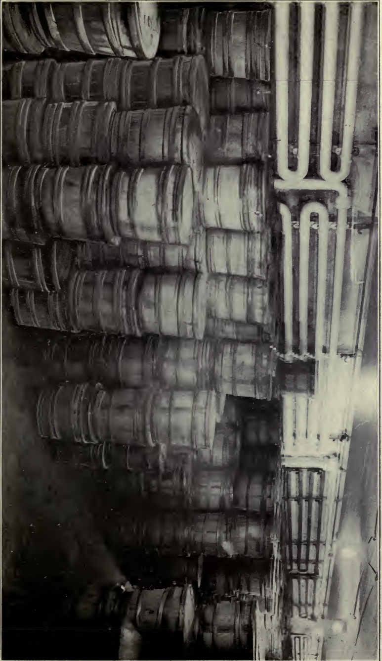
A MODERN "BUTTER BASEMENT", SHOWING REFRIGERATING PIPES THROUGH WHICH COLD AIR IS CONSTANTLY CIRCULATED
