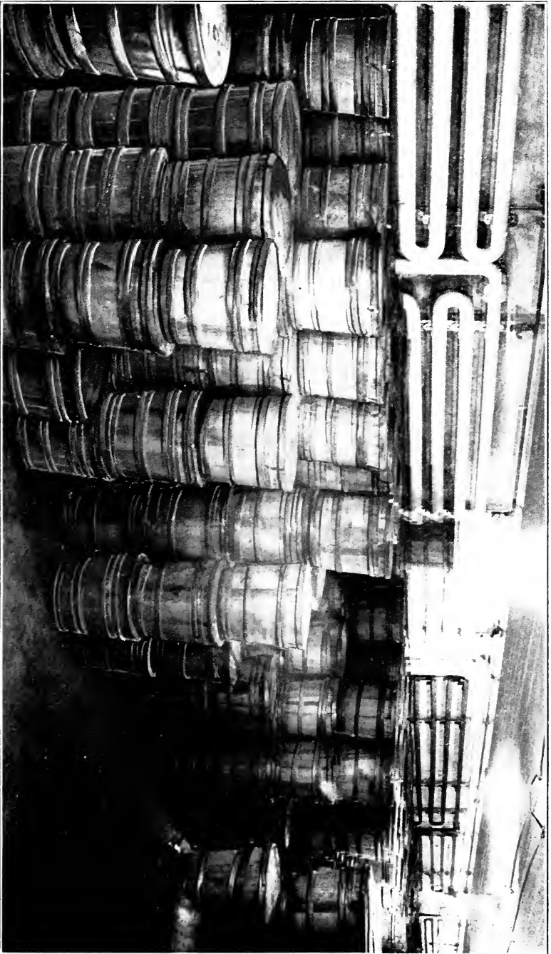
A MODERN "BITTER BASEMENT", SHOWING REFRIGERATING PIPES THROUGH WHICH COLD AIR IS CONSTANTLY CIRCULATED
