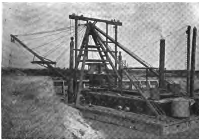
FIG. 89.—A dredge digging a ditch for irrigating an extensive area. (U. S. D. A.)
