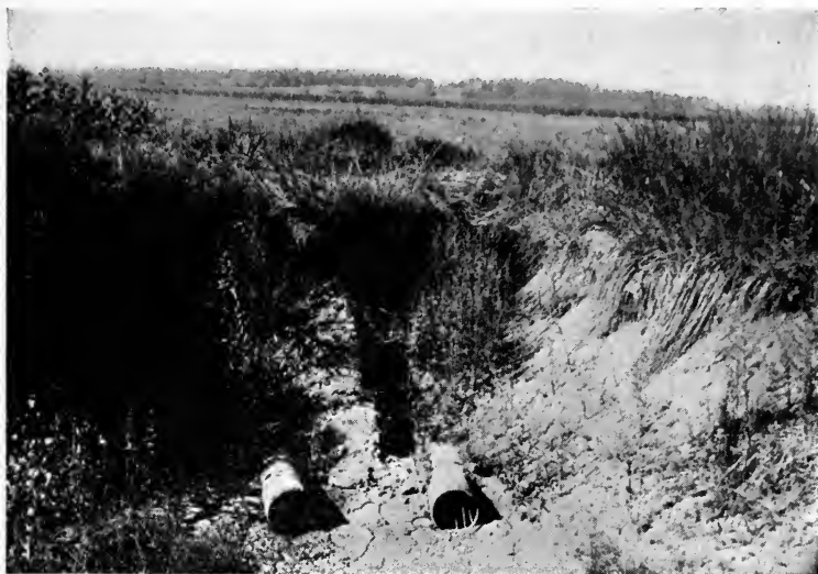
FIG. 57.—The two protected outlets to the drainage system on this marsh of 125 acres Two steel pipes screened by iron rods.
