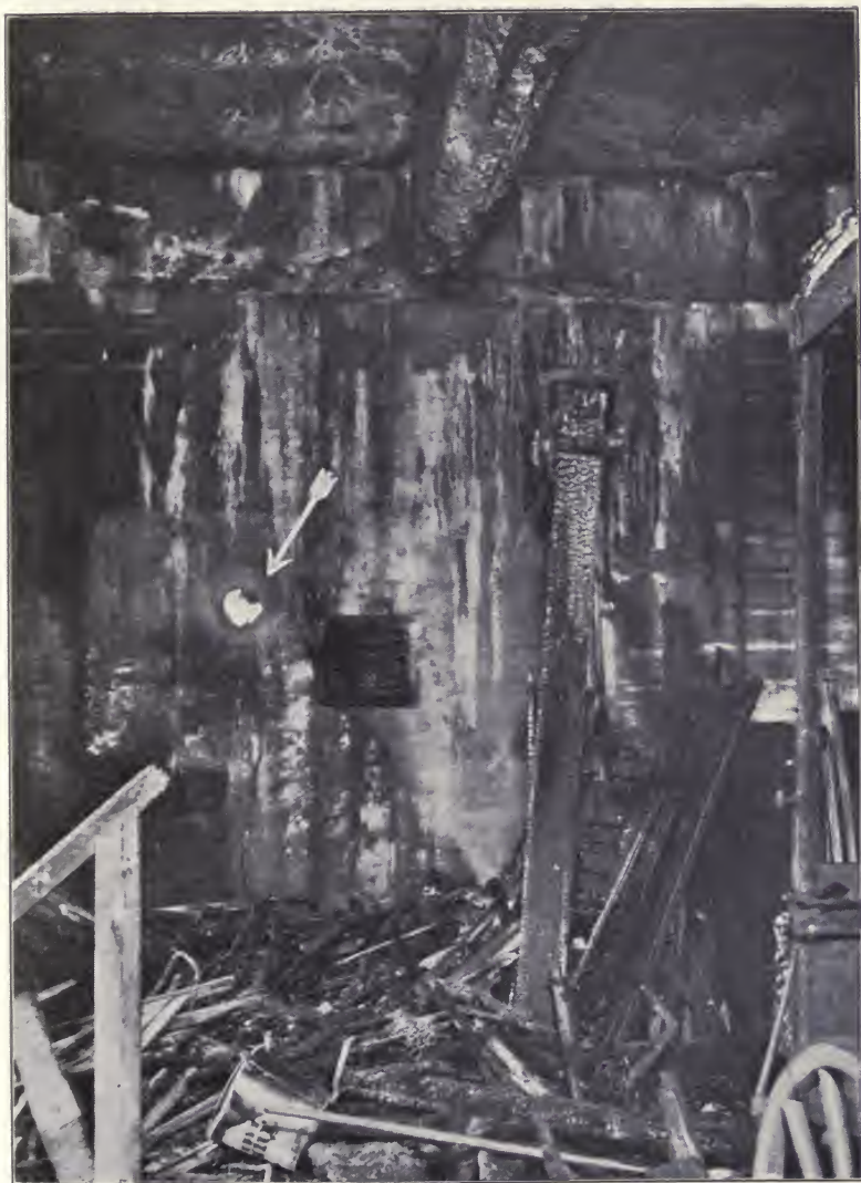
A HOLE THAT WRECKED A WAREHOUSE.
