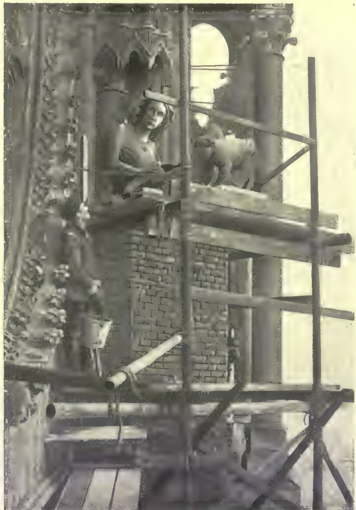
Safety-measures on the northern transept of the Rheims cathedral (According to the "Illustration" of March 23, 1918)
