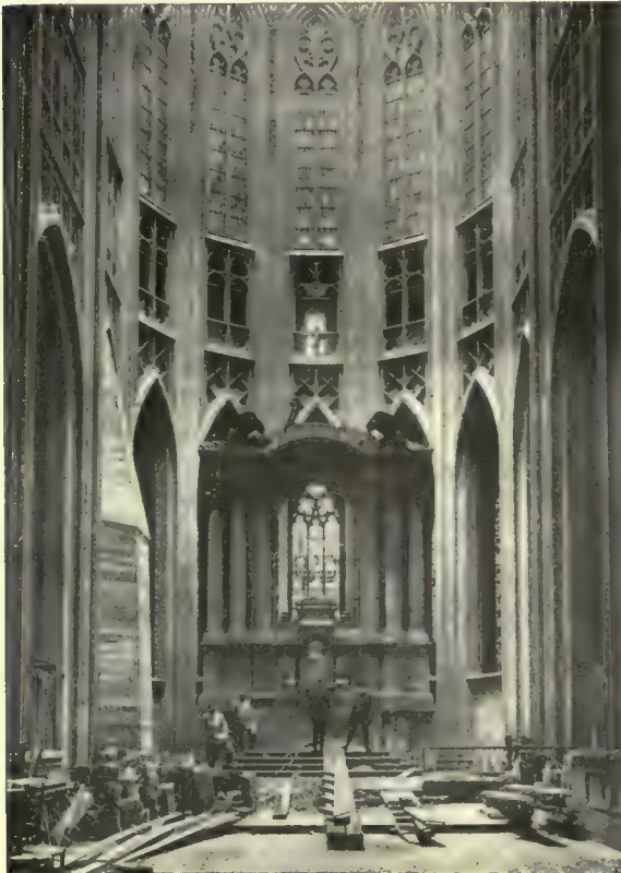
Louvain. Church of St. Peter Interior of the choir after the fire
