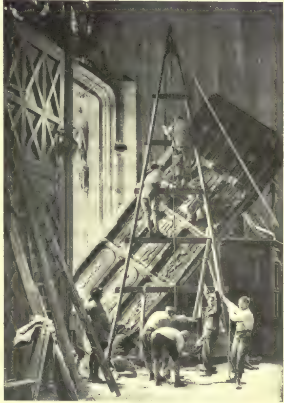
Removal of the Renaissance door of the Church of St. Vulfran, at Abbéville
