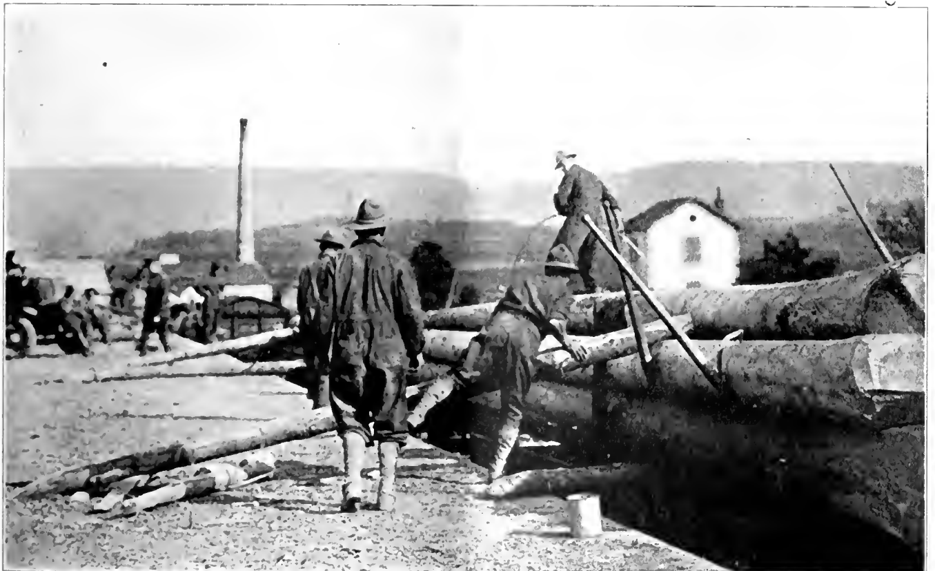
20th ENGINEERS LOADING LONG PILING FOR SHIPMENT FROM EASTERN FRANCE TO BASE PORTS ON ATLANTIC COAST TO BE USED IN DOCK CONSTRUCTION
