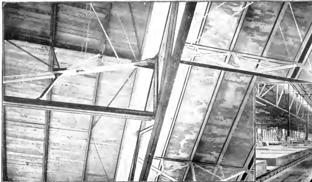
Carbosoted sheathing in place at left, and disintegrating cement ceiling at right.
