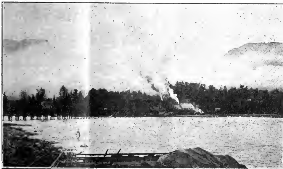
CONSTRUCTION OF STEEL BRIDGE OVER THE SUSITNA RIVER, 261 MILES NORTH OF ANCHORAGE. PRESENT END OF STEEL ON THE GOVERNMENT RAILROAD
