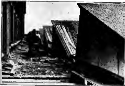
Removing decayed roof boards over textile mill — the penalty for neglecting to protect the lumber against decay before erection. (Courtesy F. J. Hoxie, Eng. Assoc. Factory Mutual Fire Ins. Co., Boston, Mass.)
