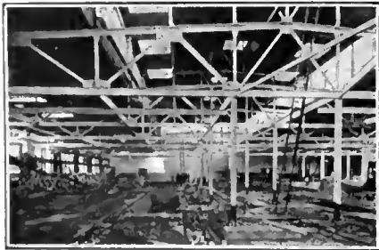
Wood Roof-Deck of Paper Mill creosoted by Open Tank process with Carbosota Liquid Creosote Oil. Dark ceiling is not a detriment.
