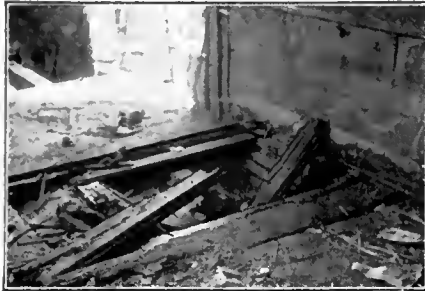
Decayed intermediate sills and flooring of freight cars.
