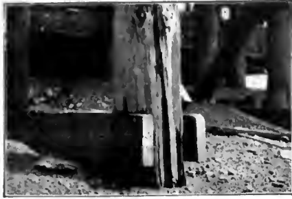
Decayed post of coal chute foundation.
