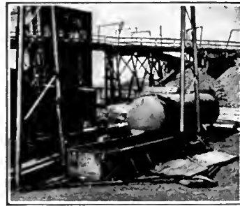
Plant of iron mine for hot and cold treatment, with 10,000 gallon storage tank for preservative. Yard crane used for handling timber.
