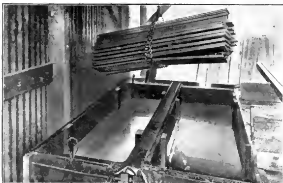
Creosoting sheathing by the Open Tank process with Carbosota Liquid Creosote Oil.
