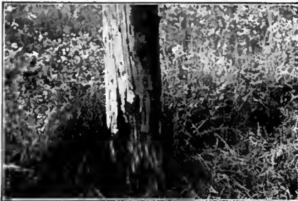
Decay is the greatest enemy of poles. Creosoting protects poles effectively.
