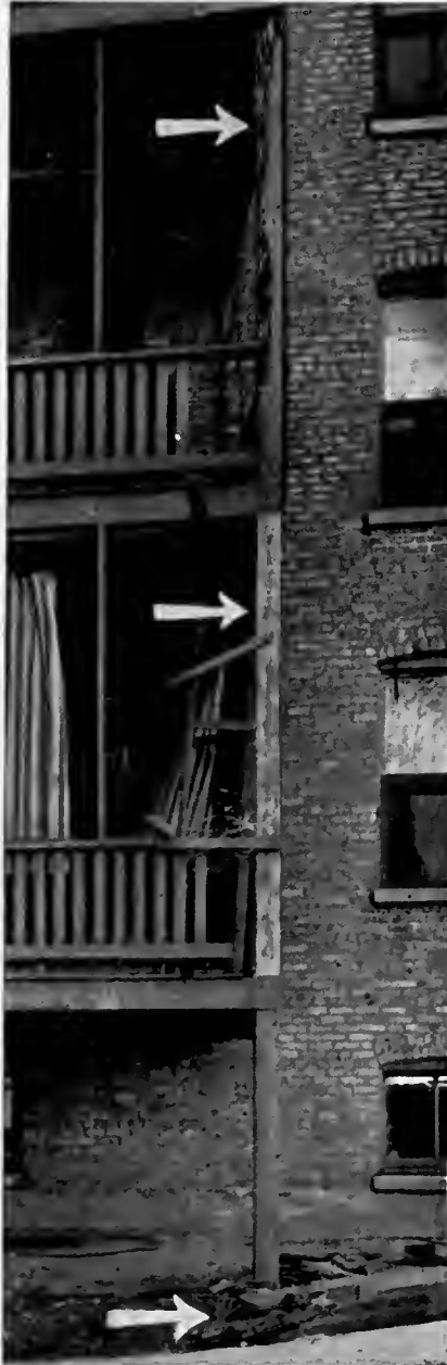
Replacement of porch columns and joists in framing of three floors is an annual occurrence at most apartment houses of this type.
