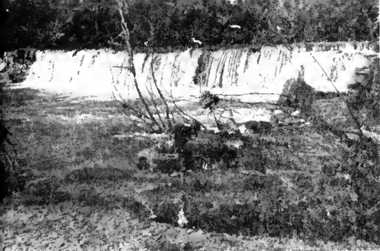
The mill dam - It has changed little since its construction by Hardeman. The top of the dam once was topped by a log to prevent debris from chipping away the top layer of stone. The canal angled away to the right.
