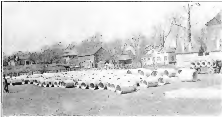
24 inch and 30 inch pipe for the sanitary effluent sewer—Batavia, N. Y. Hering & Fuller, Consulting Engineers.
