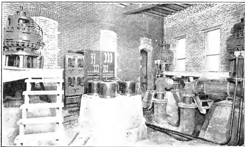
DEEP-WELL PUMPING PLANT, CHICAGO HEIGHTS, ILL.
