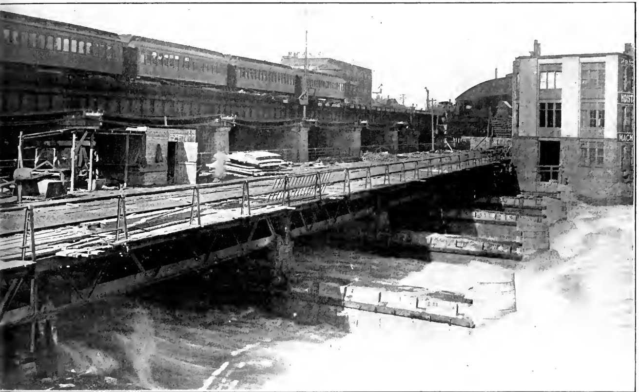
GENERAL VIEW OF OLD BRIDGE AND EXTENDED PIERS FOR NEW ONE PARTLY BUILT
