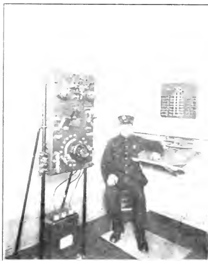
RECTIFIER AND SWITCHBOARD, FIRE ALARM SYSTEM
