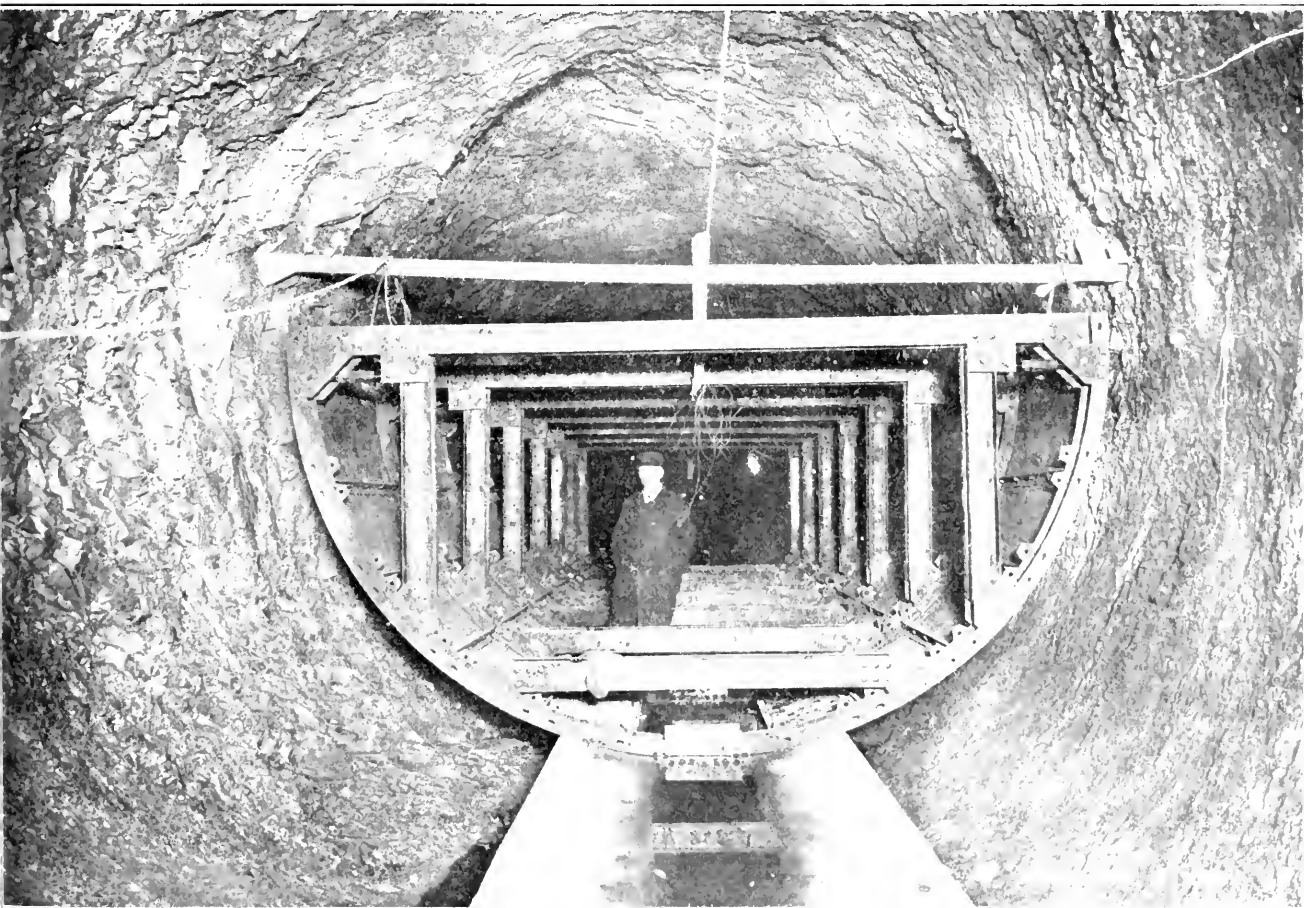
ROUNDOUT SIPHON. INVERT IN PLACE AND FORMS READY FOR SIDE WALL CONSTRUCTION
