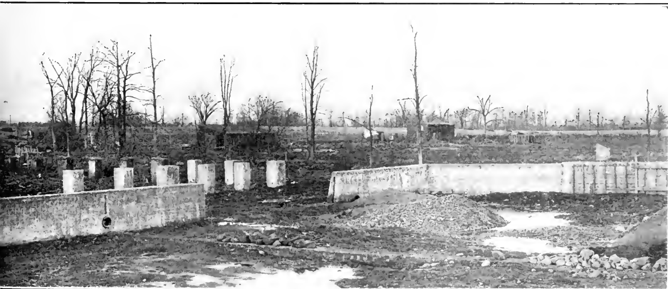
FIG. 5.—WALL OF SECOND CONTACT FILTER, AND PIERS FOR SUPPORTING FIRST CONTACT FILTER
