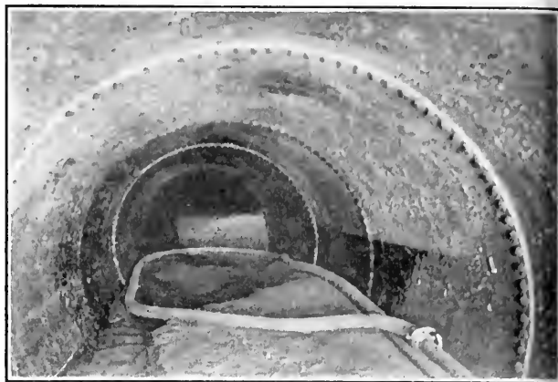
SAND PARTLY REMOVED FROM INTAKE
