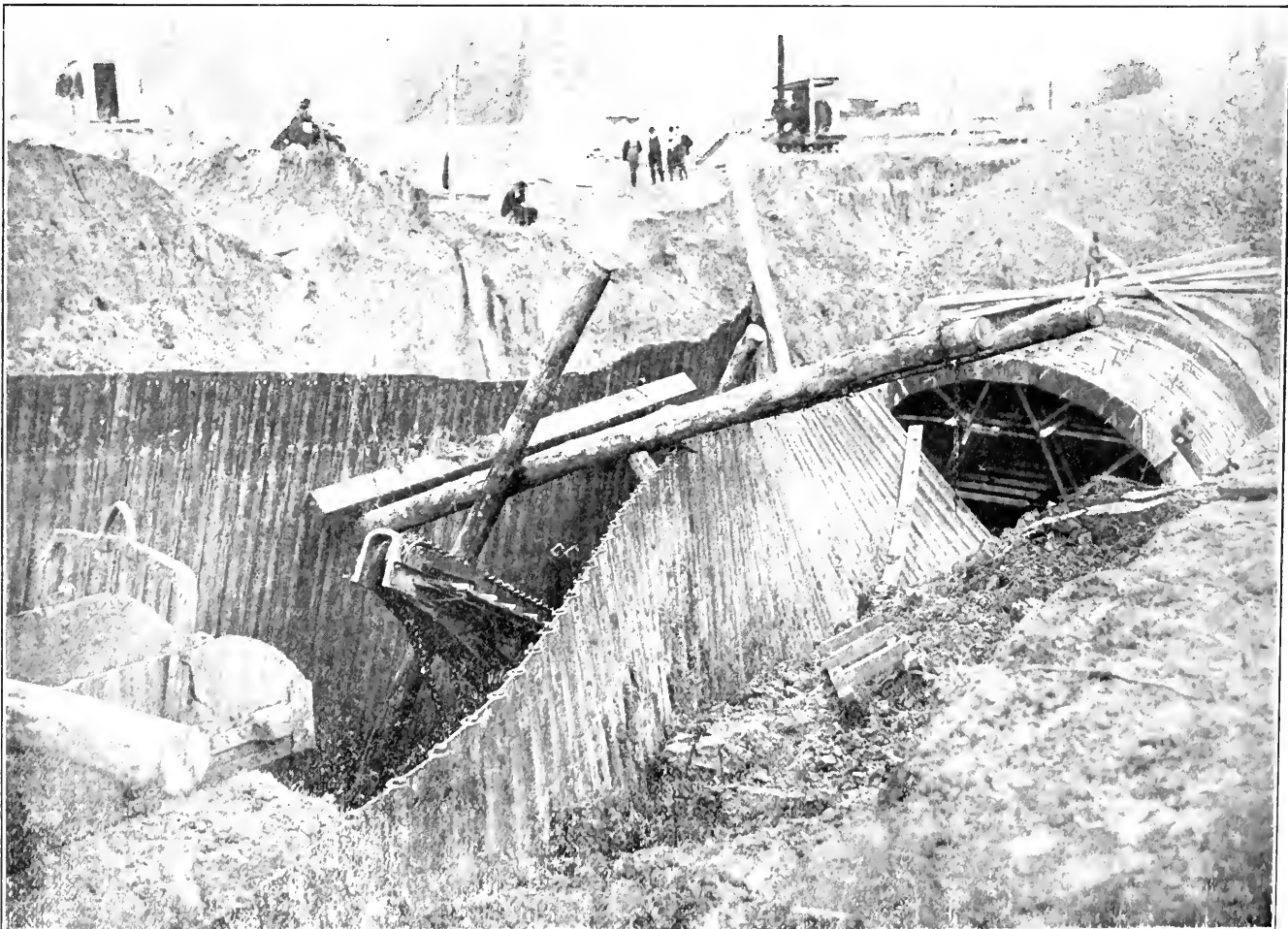
COLLAPSE OF SHEETING, 29-FOOT HARLEM CREEK SEWER Steam Shovel Protected from Earth by Steel Sheeting.
