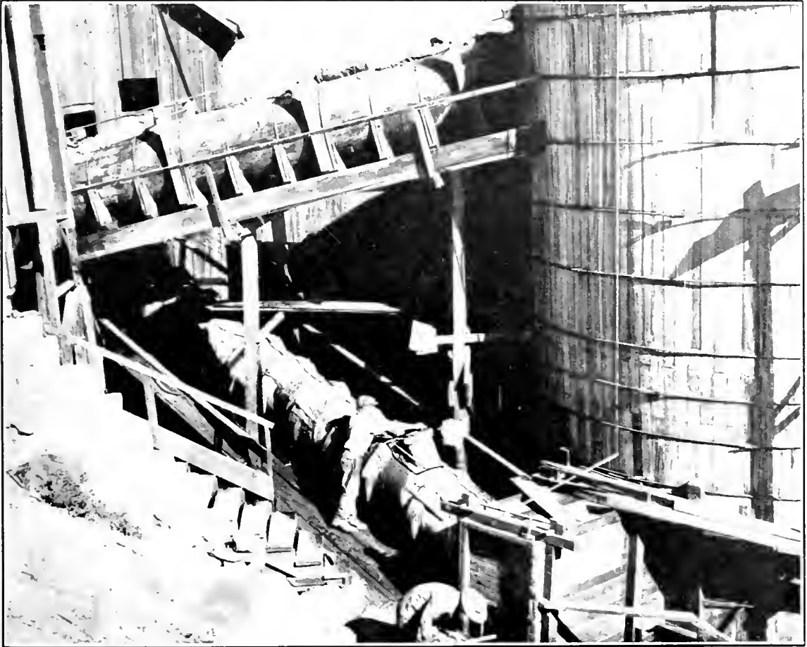
Photo No. 65. Condenser Flues—Vitrified Pipe (lower), and Wood-stave (upper),—at New Idria Mine, San Benito County.
