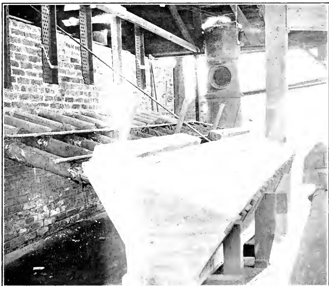
Photo No. 63. Condenser System on Johnson-McKay Retorts at Sulphur Bank Mine, Lake County.
