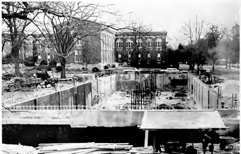
The Dana Science Laboratories under construction. New wing of library extends toward Dana building from background.
