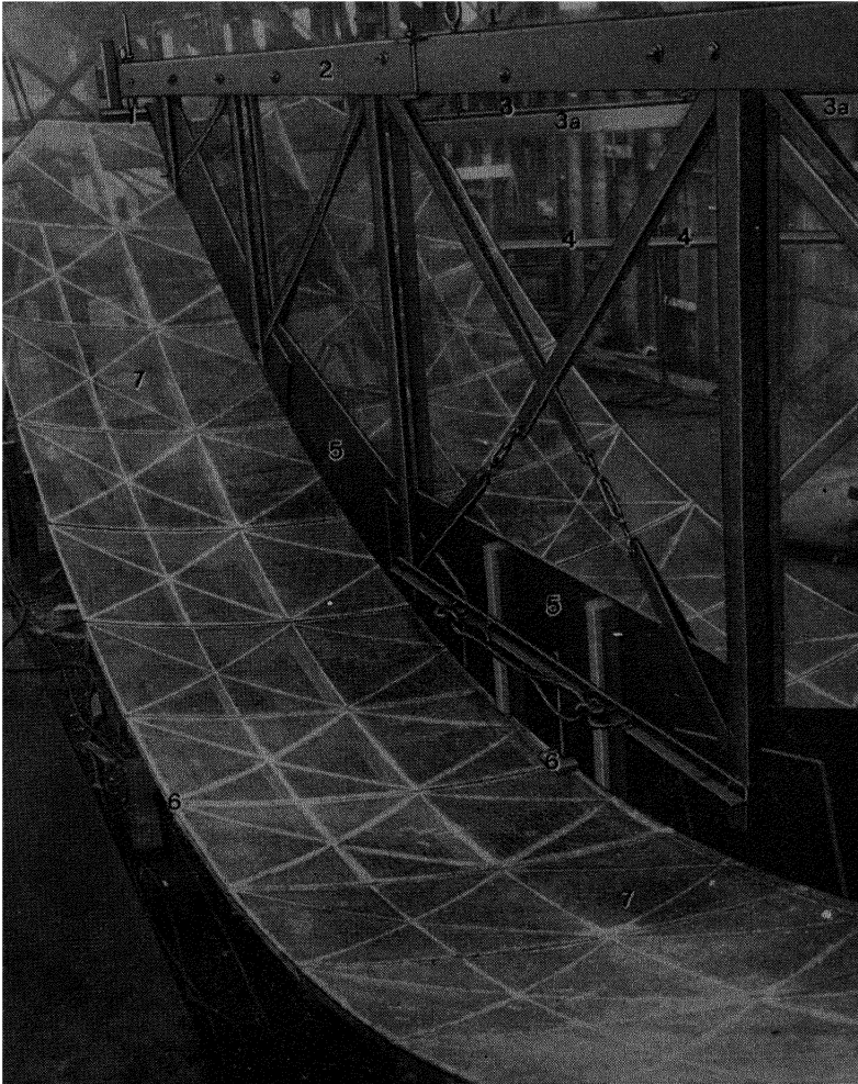
FIG. 2-4.—Reflector and template. (Courtesy of Walsh Construction Company.) 1. Template rotary truck. 2. Top chord of template truss. 3. Track. 3a. Track support. 4. Walkway. 5. Template. 6. Center support. 7. Reflector.
