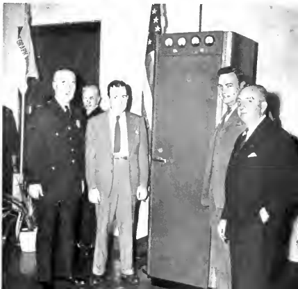
INSPECTOR BURNS (LEFT), R. A. FURLONG, L. W. SMITH AND AL JOSEPHSEN OF RCA STAND IN FRONT OF 250-WATT FM TRANSMITTER AT BROOKLYN POLICE HEADQUARTERS.
