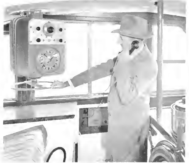
Radiomarine direction finder installed in the wheel-house of the yacht Seaquester .
