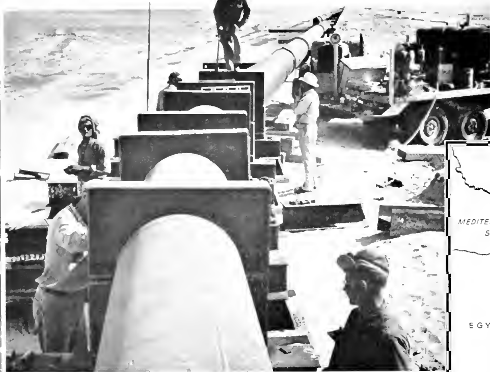
Left: Section of Tapline conduit which carries daily flow of 300,000 barrels of oil over 1,000 mile route shown below.
