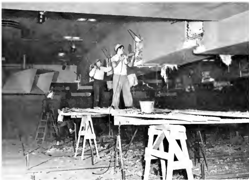
IN REVAMPING NBC'S FAMOUS CONCERT STUDIO 8-H, WORKMEN REMOVE CEILING BEAMS TO MAKE WAY FOR A STEEL OVERHEAD CONSTRUCTION.
