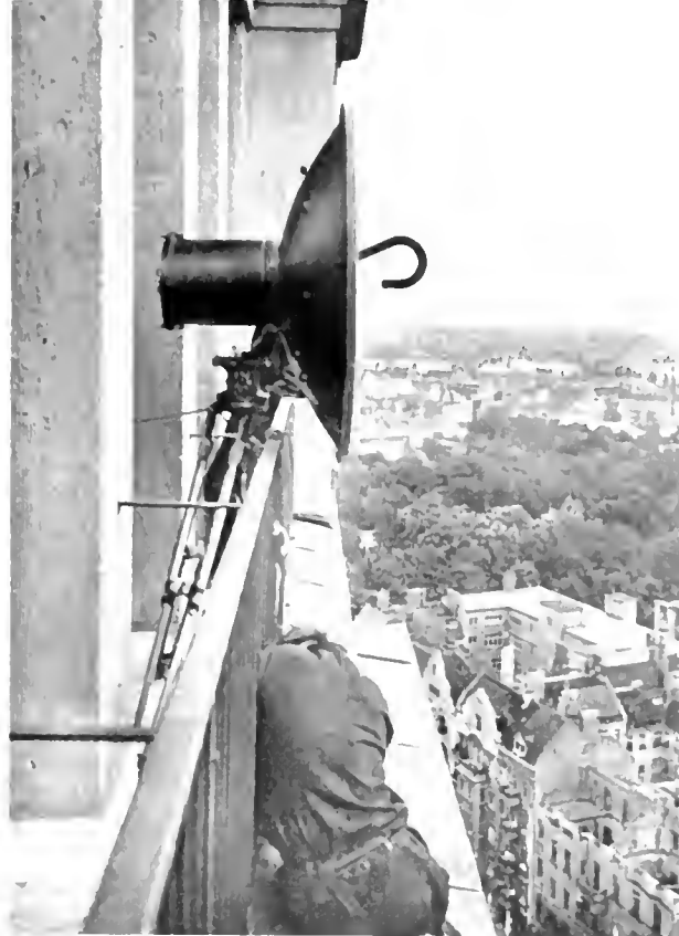
One of the two microwave relay units used in the Berlin telecasts was mounted on the side of the City Hall tower, one of the highest points in the area.
