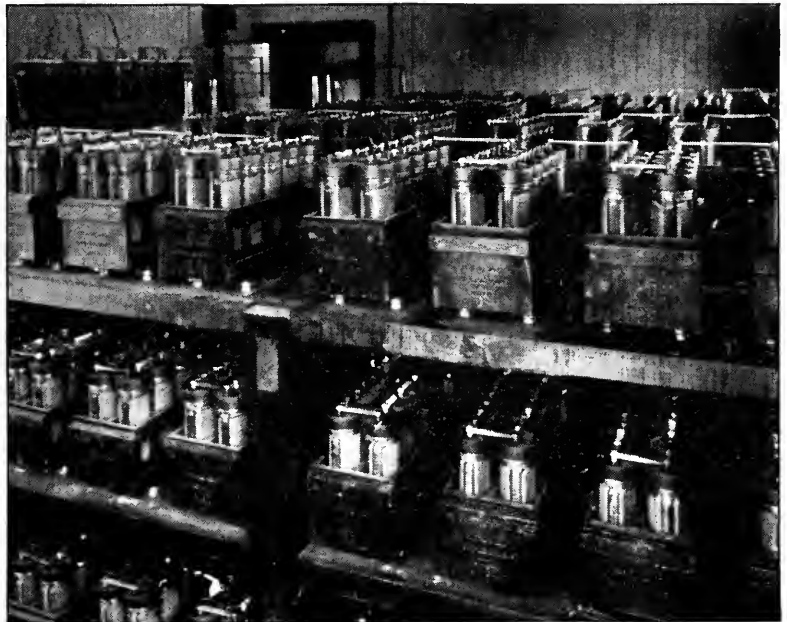
A FEW OF THE 1,400 BATTERIES THAT SUPPLY THE JUICE FOR WTAM Station of the Willard Storage Battery Company in Cleveland, Ohio
