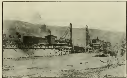
WASHOUT ON THE LINE—BRIDGE GONE OUT.
