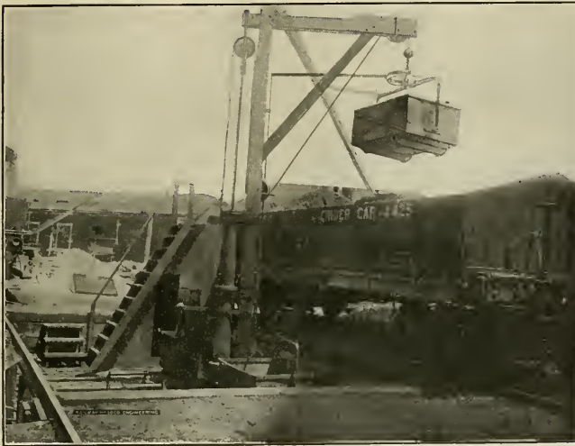
FIG. 3. ASH BUCKET OVER CAR READY FOR DUMPING.
