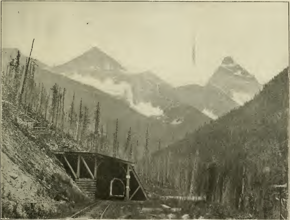
SNOW SHED, WITH SPLIT FENCE ABOVE, IN THE SELKIRK MOUNTAINS, ON THE CANADIAN PACIFIC RAILWAY.
