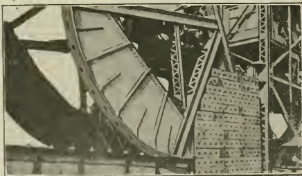
ROLLER OF BRIDGE AND COUNTERWEIGHT—C. R. R. OF N. J., NEWARK BAY.
