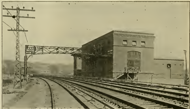
N. Y. C., SUB-STATION NO. 3, SHOWING POLE AND OVERHEAD CONSTRUCTION (Courtesy of Street Railway Journal)
