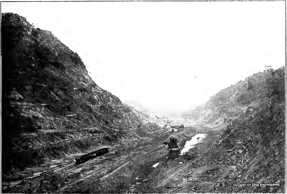
CULEBRA CUT, THE LARGEST EXCAVATION ON THE ROUTE OF THE PANAMA CANAL.
