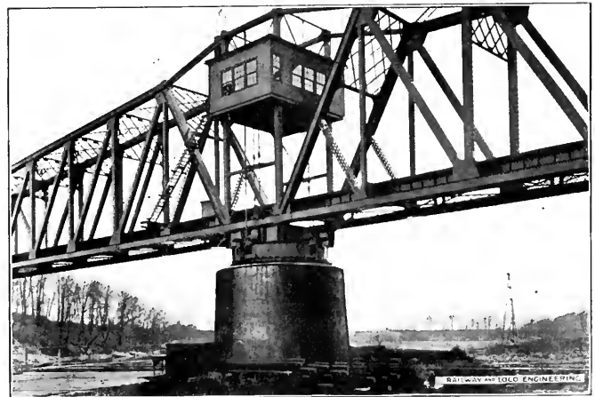
EXAMPLE OF SWING BRIDGE SHOWING TURNABLE AND CENTER PIER. BRIDGE MUST OPEN FULLY FOR EVERY VESSEL.
