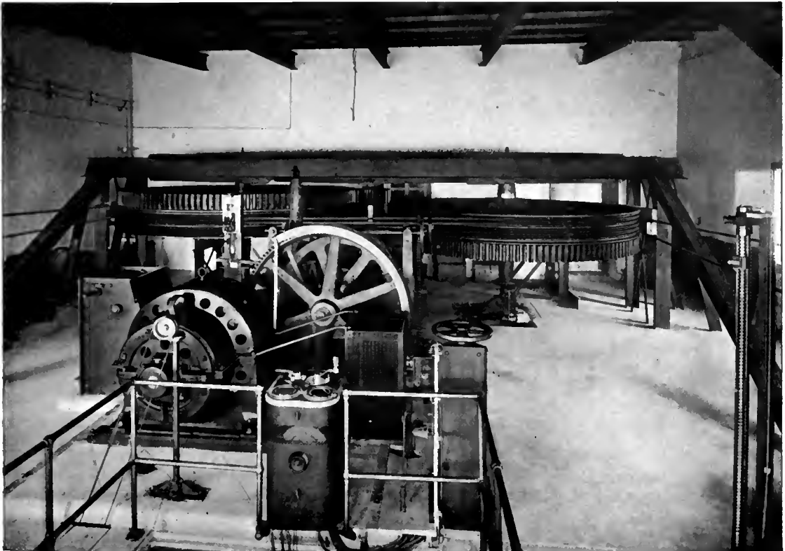
INTERIOR OF THE DRIVING STATION, WETTERHORN AERIAL RAILWAY. Showing the two great winding drums driven by a 45-horse-power electric motor.
