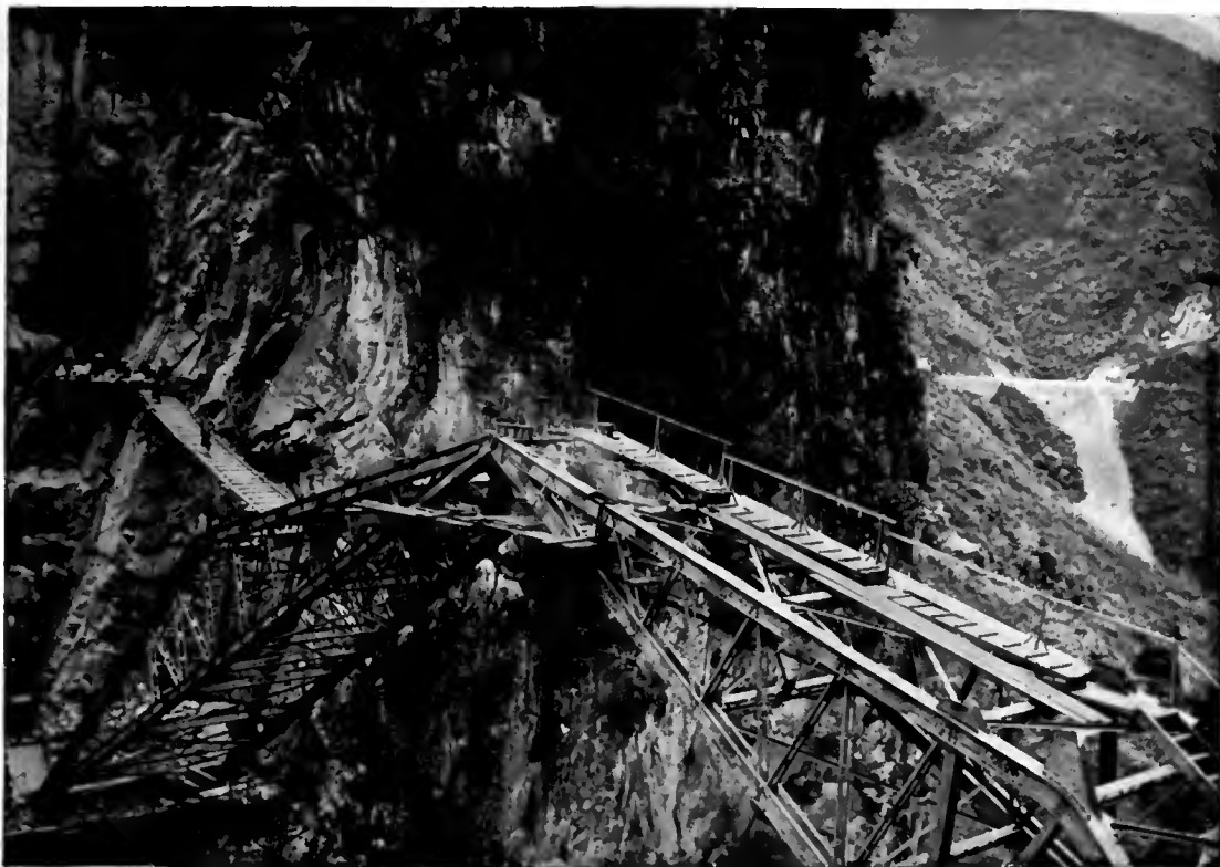
THE BASCULES OF THE FAUX NAM-TI BRIDGE, CONNECTED, SHOWING TEMPORARY GANG PLANKS.
