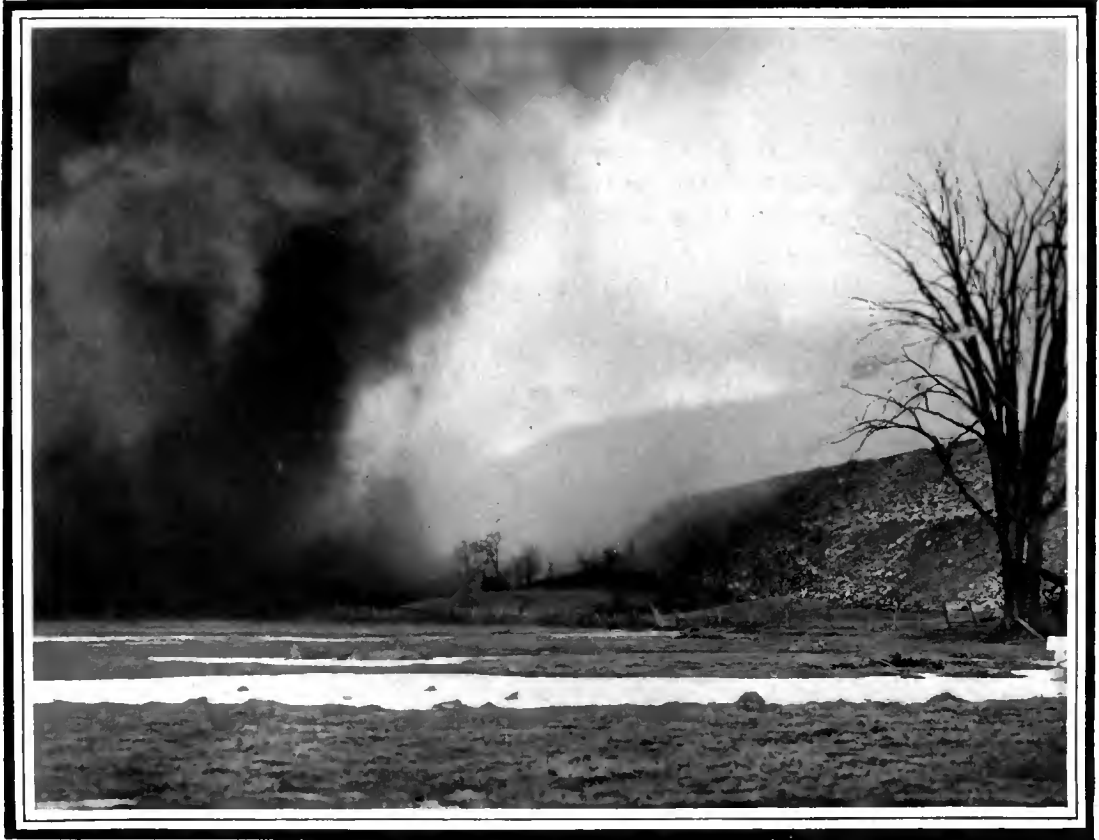
A 16½ TON BLAST ON THE LACKAWANNA CUT-OFF. 5,000,000 lb. of dynamite were used in this reconstruction work.
