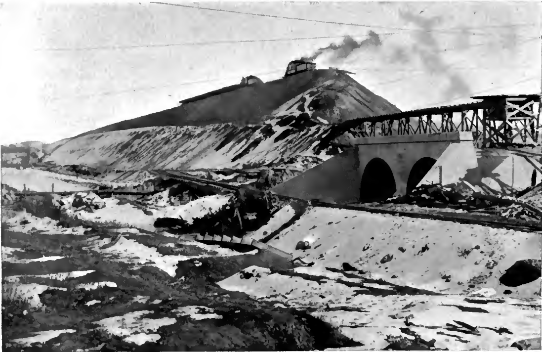
BUILDING UP THE PEQUEST FILL ON THE LACKAWANNA CUT-OFF. This enormous embankment absorbed over 6,600,000 cubic yards of material.
