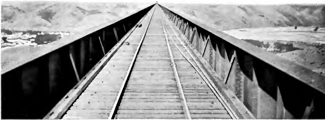
LOOKING ALONG THE DECK OF LETHBRIDGE VIADUCT. Showing girders rising above the rails and forming a trough for traffic.
