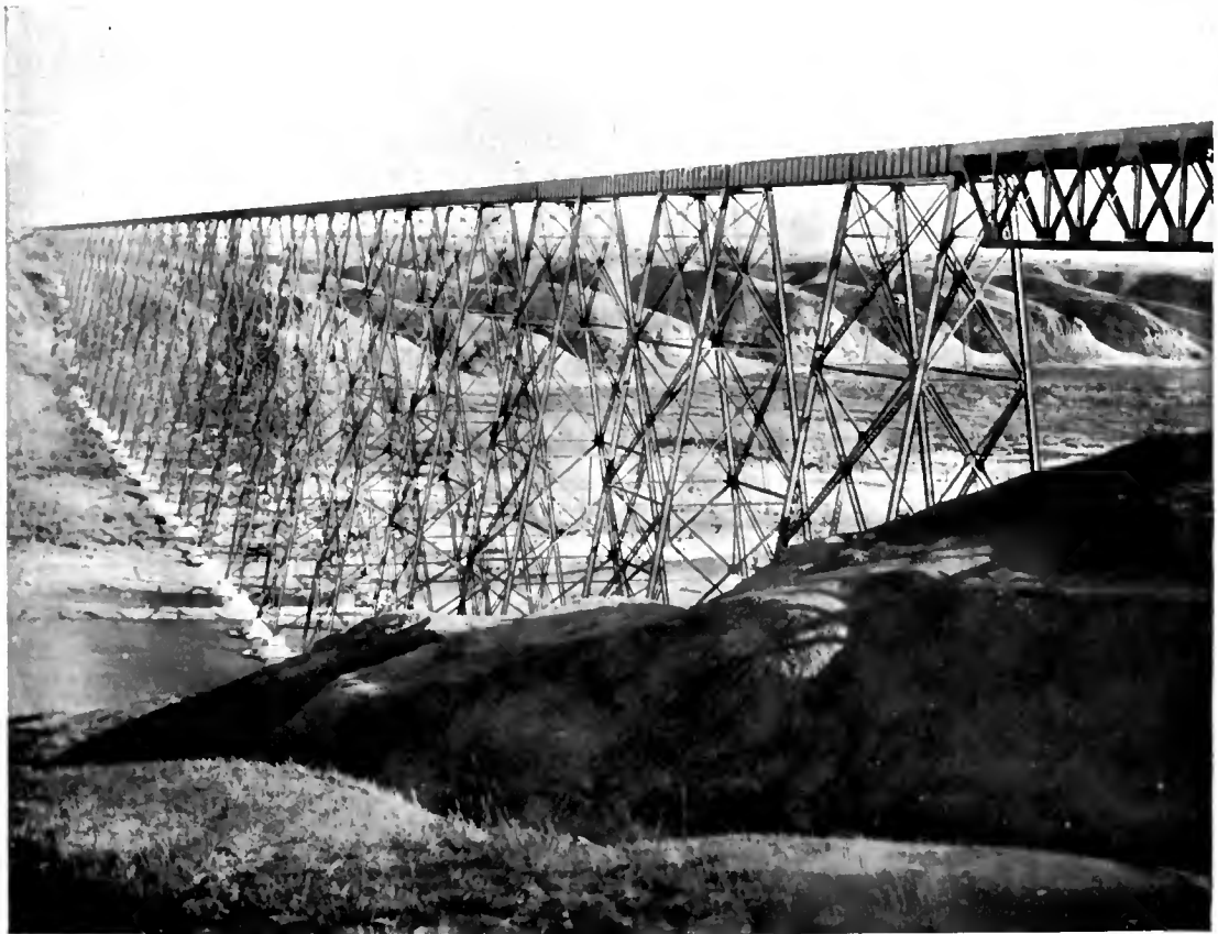
THE LETHBRIDGE VIADUCT, ALBERTA: IT IS 5,327 FEET 7½ INCHES LONG AND 314 FEET HIGH.
