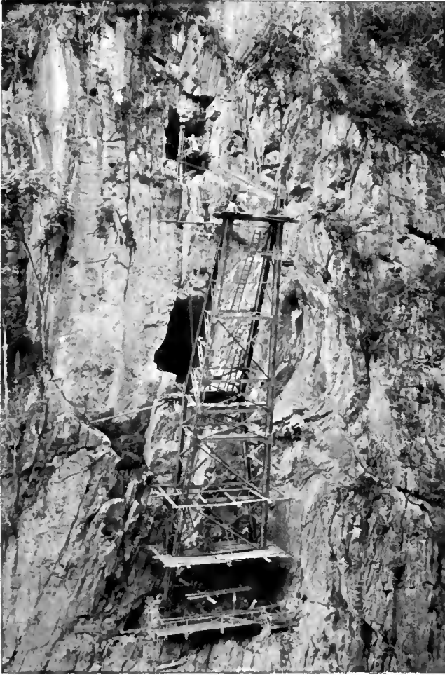
BUILDING A BASCULE OF THE FAUX NAM-TI BRIDGE UP ONE OF THE CLIFF FACES.
