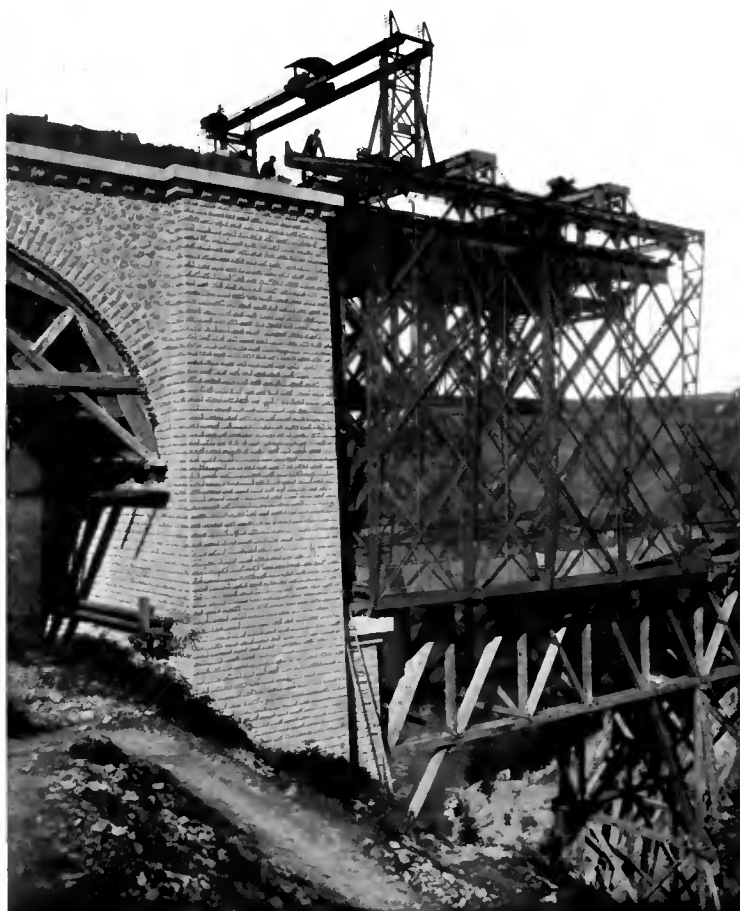
COMMENCING THE STEELWORK ON ONE OF THE SHORE SPANS: SHOWING THE WIRE-NETTING ENCLOSED TRAVELLER.
