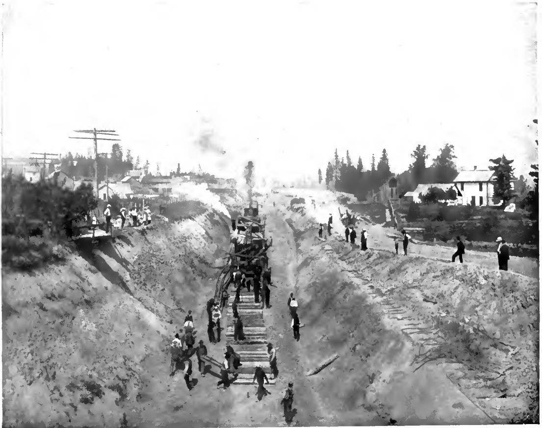
LAYING THE METALS AT THE RATE OF FIVE MILES A DAY. The track-layer at work on the Chicago, Milwaukee and Puget Sound Railway.
