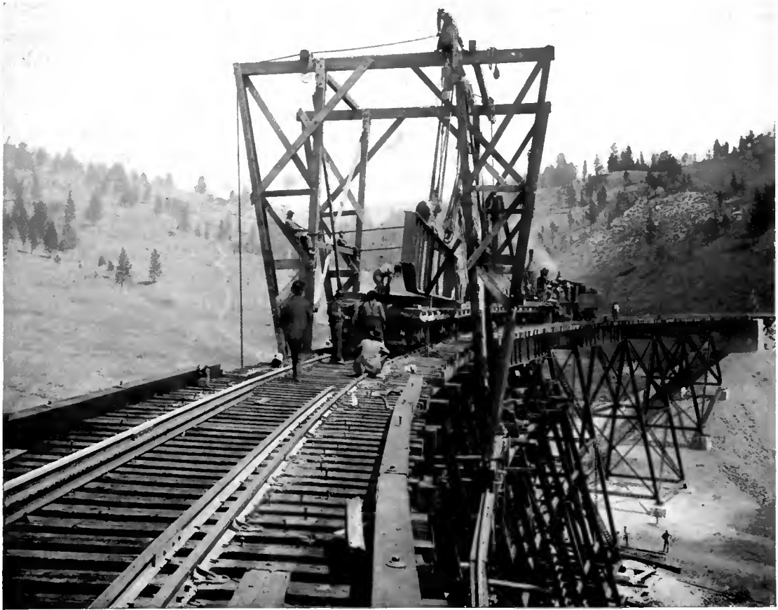
REBUILDING IN STEEL THE OLD TIMBER TRESTLE ACROSS GREENHORN GULCH IN THE ROCKY MOUNTAINS.
