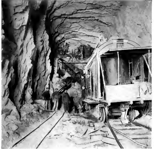
THE MECHANICAL SHOVEL WORKING IN A TUNNEL AND DRIVEN BY COMPRESSED AIR.
