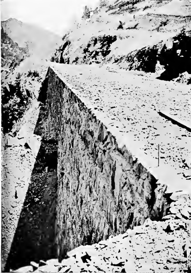
MASONRY WALL THROWN ACROSS A RIFT IN THE MOUNTAIN, AND FILLED BEHIND TO PROVIDE A SHELF TO SUPPORT THE METALS.
