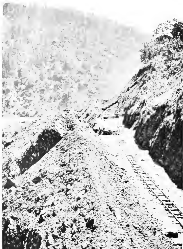
DRIVING THE PERMANENT WAY THROUGH THE RUGGED MOUNTAINS 40 MILES EAST OF OROVILLE, CALIFORNIA.
