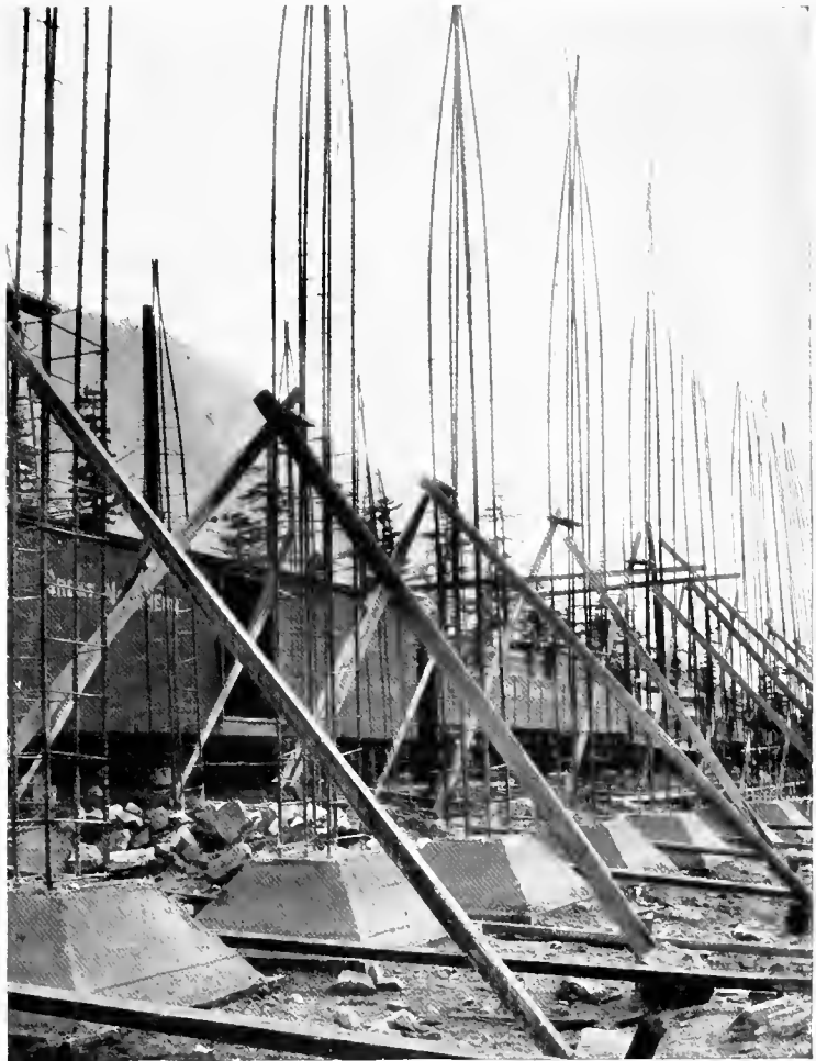
THE NEW CONCRETE SNOW-SHEDS, CASCADE SUMMIT. The reinforcing steel for the posts on the lower side of the line.
