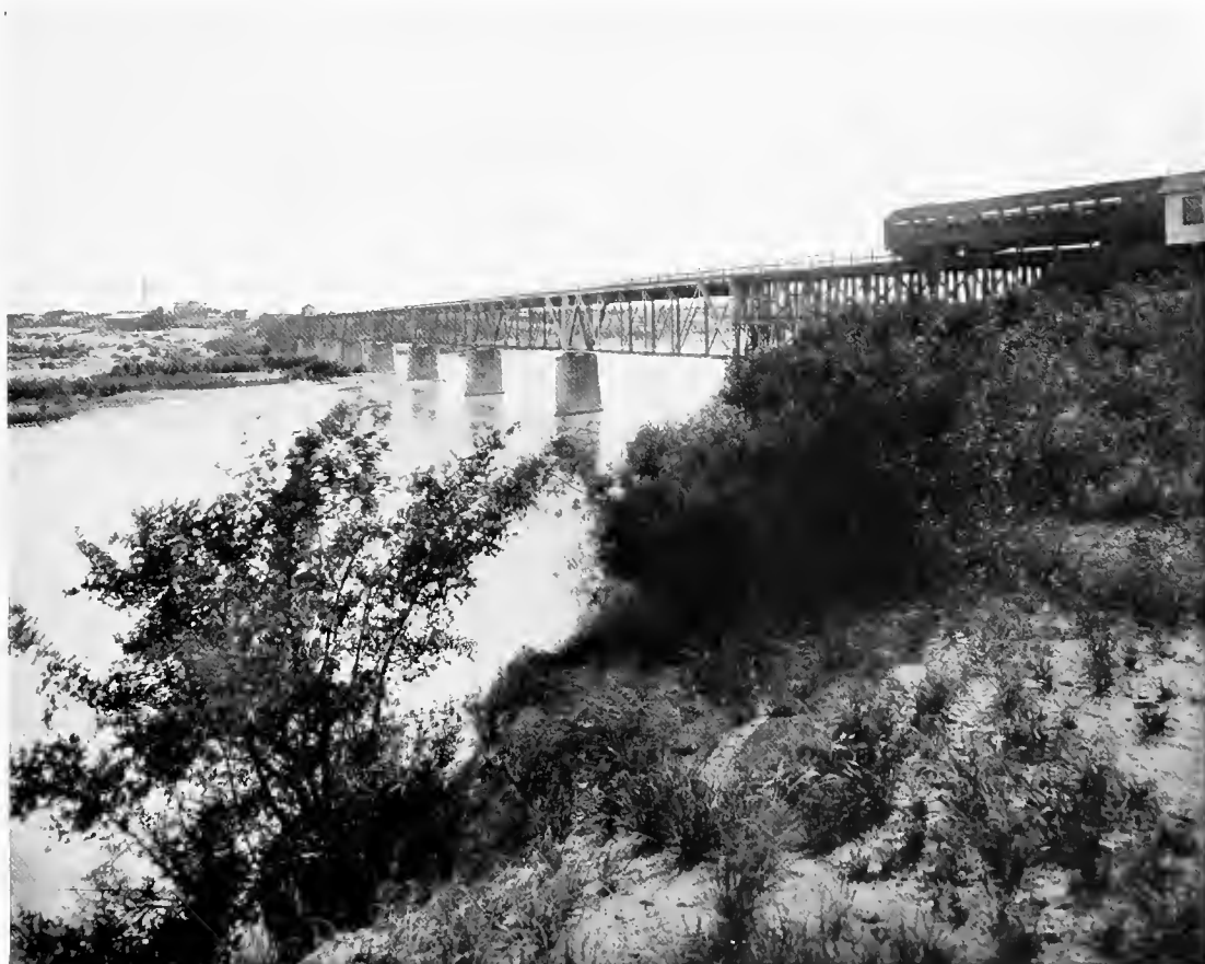
LAREDO BRIDGE, BETWEEN LAREDO, TEXAS, U.S.A., AND NUEVA LAREDO, MEXICO. It comprises six spans each of 175 feet, with an approach at each end 65 feet in length.
