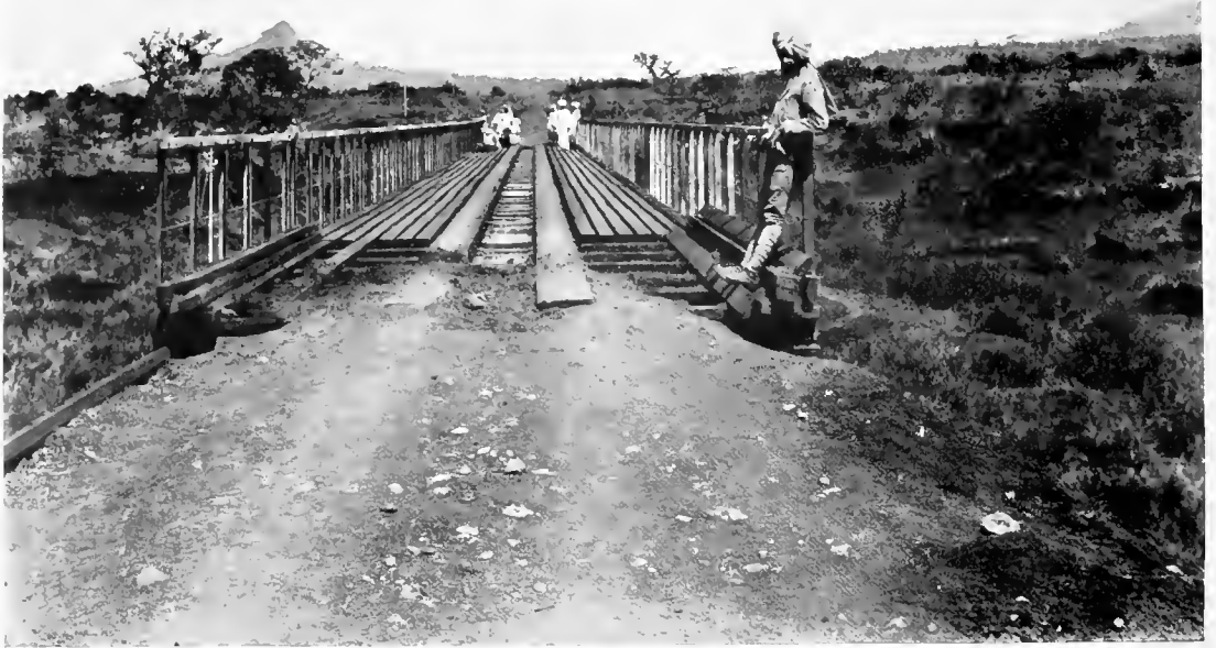
THE MAKING OF THE UGANDA RAILWAY: READY FOR THE RAILS. A bridge completed and the grade finished to foundation level.
