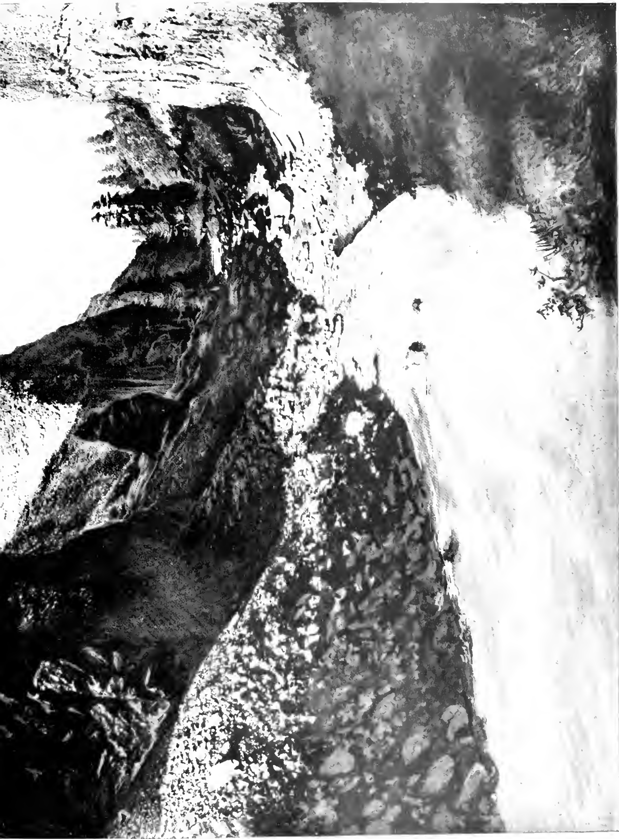
SETTING THE LAST PIECE OF STEEL TO COMPLETE THE CROOKED RIVER CANYON BRIDGE.
