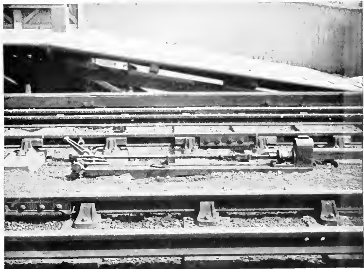
THE AUTOMATIC STOP WHEREBY TRAINS ARE BROUGHT TO A STANDSTILL INDEPENDENTLY OF THE MOTOR IF THE SIGNALS ARE AT DANGER.
