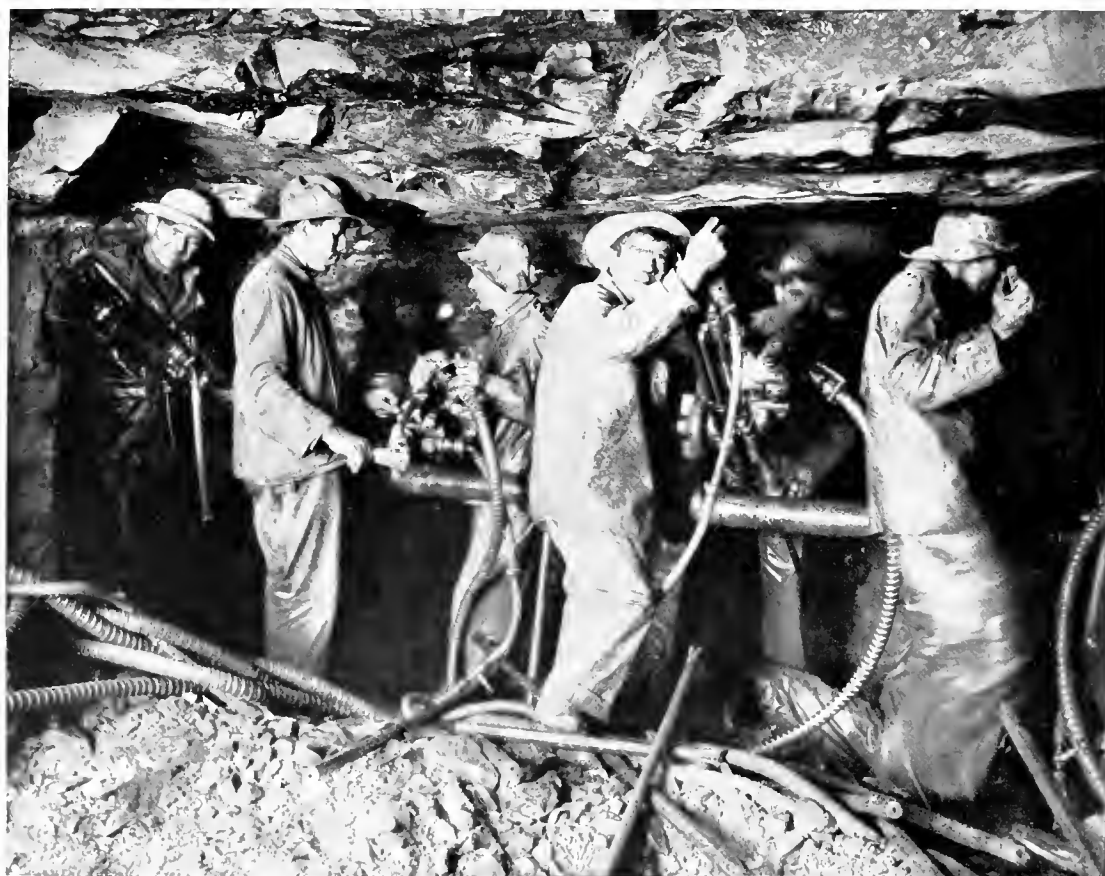
Photograph by permission of the Canadian Northern Railway. DRIVING THE TUNNEL THROUGH MOUNT ROYAL TO GIVE THE CANADIAN NORTHERN ACCESS TO MONTREAL.
