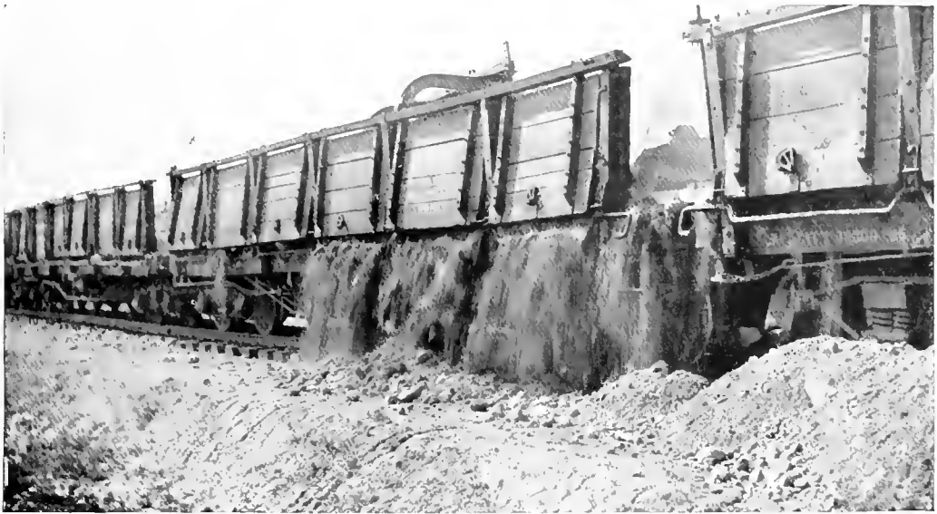
THE SPOIL FALLING FROM THE TRUCKS AS THE UNLOADER IS PULLED ALONG. The sides of the Truck are top-hinged doors.
