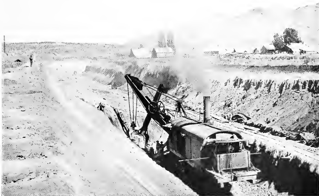
STEAM SHOVEL EXCAVATING THE BOTTOM LEFT OF THE BECKWORTH TUNNEL APPROACH, THE SUMMIT LEVEL OF THE WESTERN PACIFIC RAILWAY, 4,956 FEET ABOVE THE SEA.
