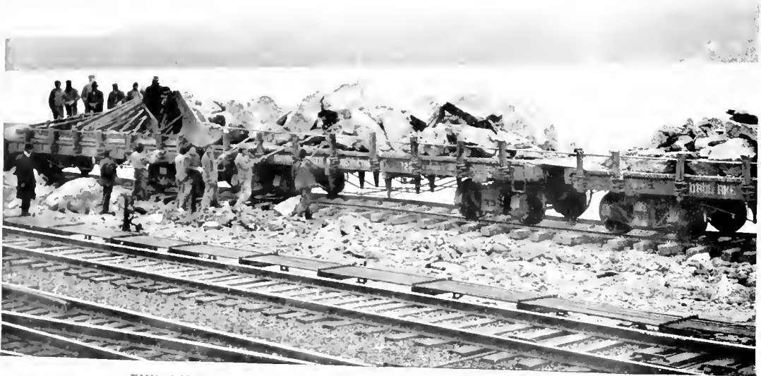
THE LIDGERWOOD UNLOADER DUMPING ROCK FROM A TRAIN. Showing plough and hauling rope.
