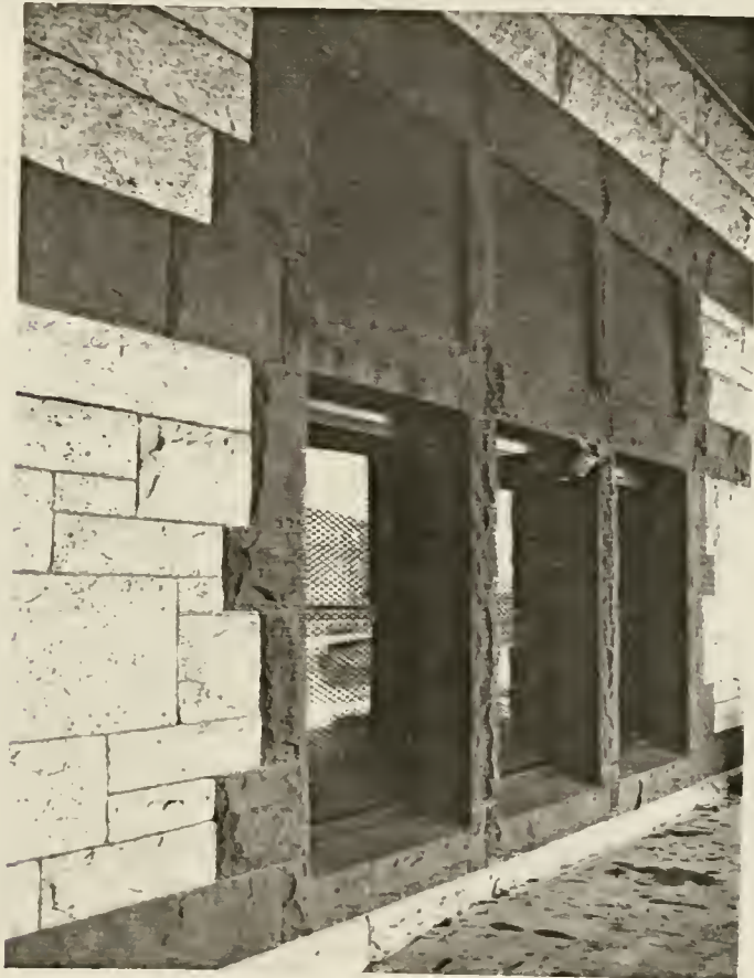
FIGURE 42: Connecticut River Railroad Station, cement-block filled windows.
