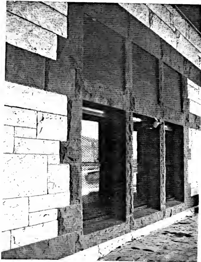
FIGURE 42: Connecticut River Railroad Station, cement-block filled windows.
