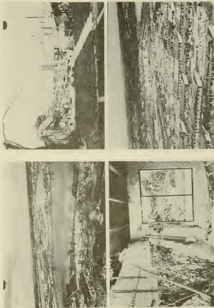
C-3. Upper left - Streaks of damage in Naranja Lakes development; upper right - home where a widow stayed with her cats that she could not take to a shelter and was killed by debris; lower left - shows concrete tie beam, but no tie columns, the primary reason for the catastrophic failures in the CBS buildings where they were not present; lower right - other streaks in Naranja Lakes area which also show a well engineered building (school) that withstood the force of the hurricane.
