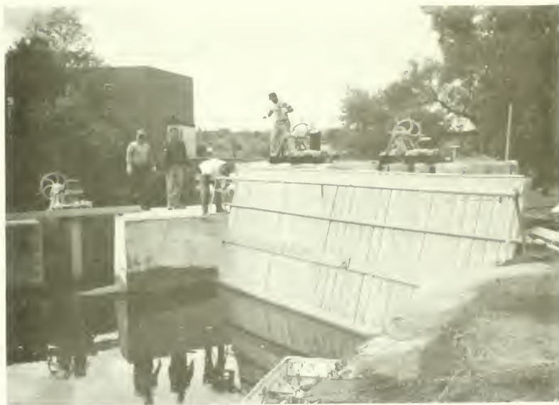
Repair to Penstock Opening wooden grate (Pleasant Street) Public Works Employees: (l-r) Ted Mikolyski, Jay Perkins, George Sturgis & Joe Pelchat
