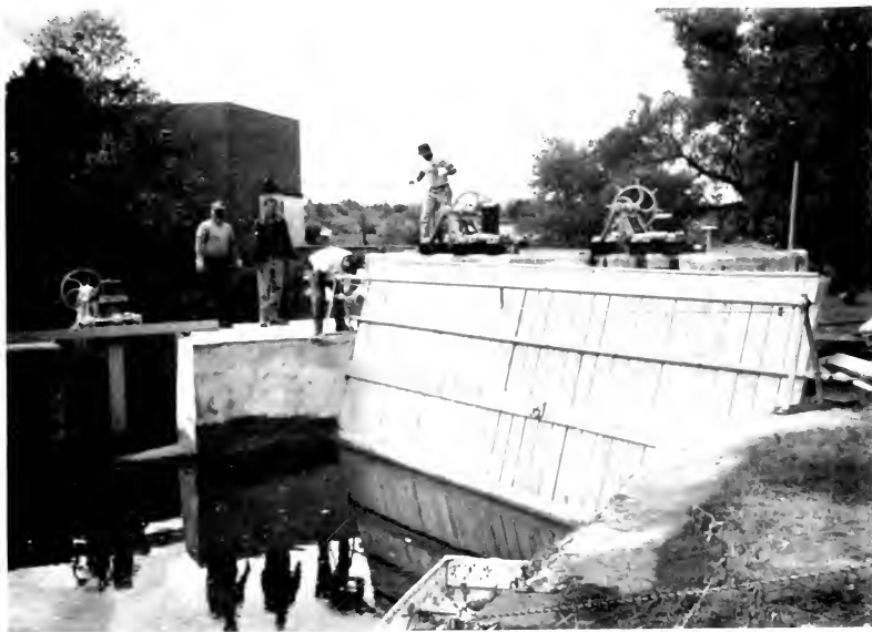
Repair to Perstock Opening wooden grate (Pleasant Street) Public Works Employees: (l-r) Ted Mikolycki, Jay Perkins, George Sturgis & Joe Pelchat
