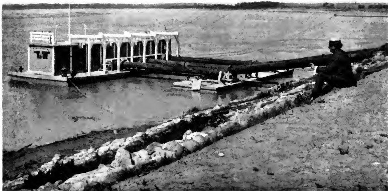
PUMPING BARGE AT LOW WATER ON THE MISSOURI RIVER AT WILLISTON WILLISTON PROJECT, NORTH DAKOTA
