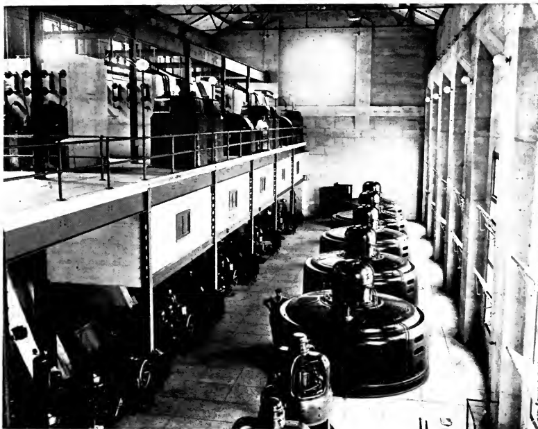
INTERIOR OF MINIDOKA HYDRO-ELECTRIC POWER-HOUSE MINIDOKA PROJECT, IDAHO
