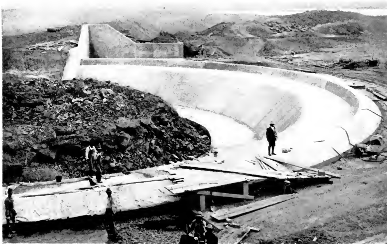
SPILLWAY AT HEAD OF WASTE CHANNEL, NORTH END OF BELLE FOURCHE DAM BELLE FOURCHE PROJECT, SOUTH DAKOTA
