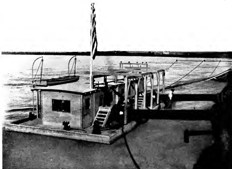
PUMPING BARGE AT HIGH WATER, WITH SINGLE LENGTHS OF DISCHARGE PIPES BETWEEN THE BALL-JOINTS ON THE BARGE AND BANK OF THE MISSOURI RIVER WILLISTON PROJECT, NORTH DAKOTA
