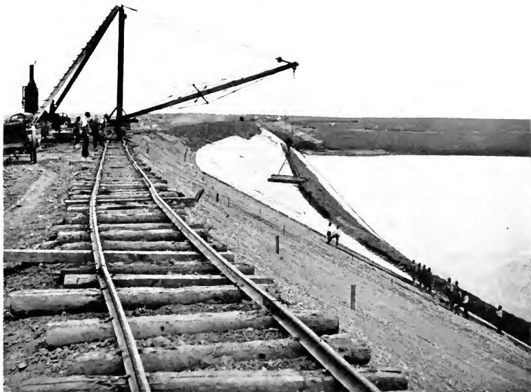
PLACING THE CONCRETE BLOCKS ON UPSTREAM FACE OF BELLE FOURCHE DAM BELLE FOURCHE PROJECT, SOUTH DAKOTA
