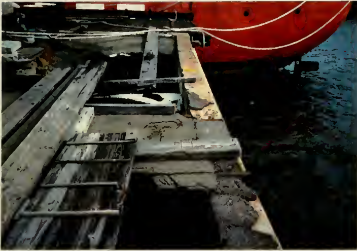
Sinkholes at Bulkhead
