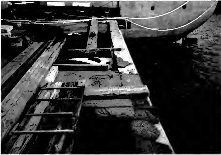
Sinkholes at Bulkhead
