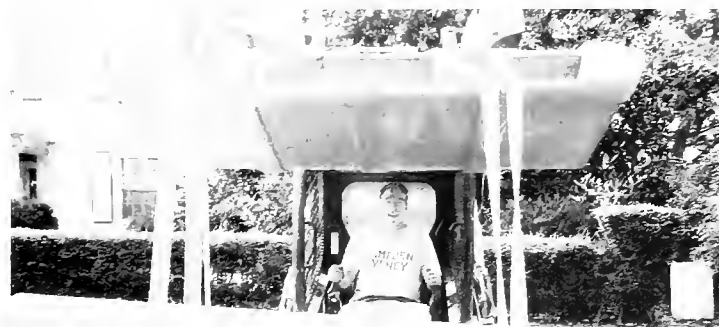
Brian Dyer '83 placing the granite curbing for the driveway of his house, which was recently renovated by David King '83.
