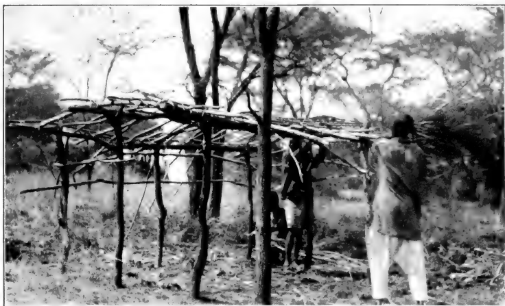
CONSTRUCTING ONE OF THE STOREHOUSES OR "CACHES" IN WHICH WE HAD TO LEAVE OUR SURPLUS GOODS
