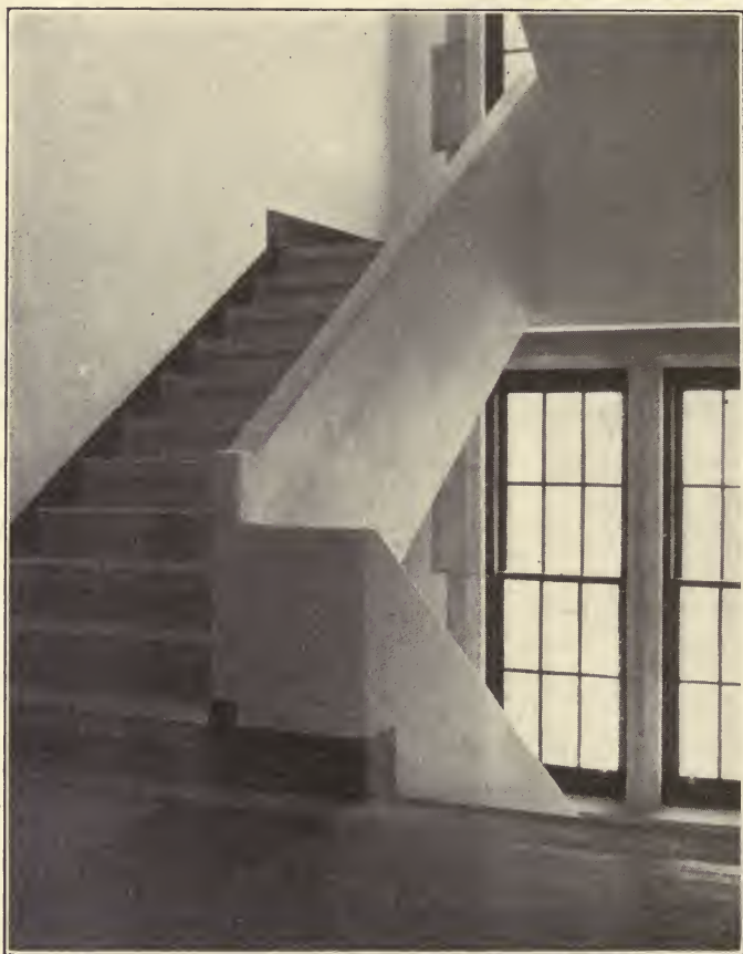
FIGURE 145. MONOLITHIC CONCRETE STAIRS AND RAIL, CAST IN ONE PIECE THREE STORIES HIGH. CONCRETE WAS RUBBED WITH CARBORUNDUM AND PAINTED.
