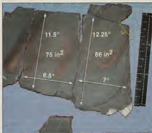
Figure 3.8-11. Three large pieces of debris from the panel face sheet were lodged within the hollow area behind the RCC panel.
