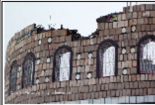
The effects of indiscriminate shelling on the houses in the town of Lauder- Abyan in 20.08.2010
