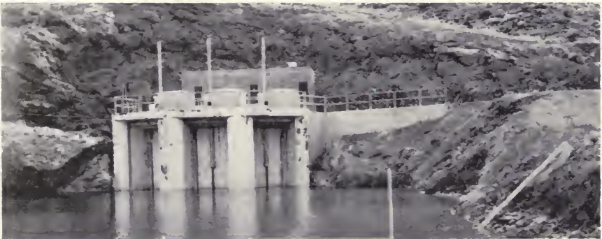
Outlet gates at Copper Basin
