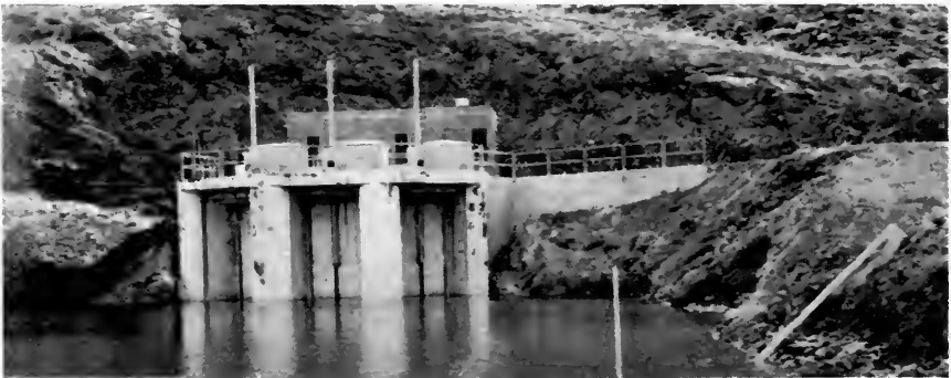
Outlet gates at Copper Basin
