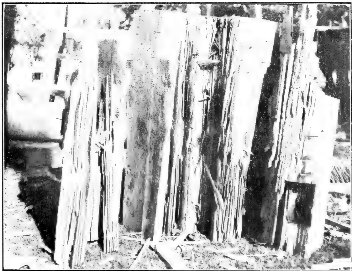
Plate 15. Fig. 2. Timbers destroyed by Termites or White Ants in Honolulu.
