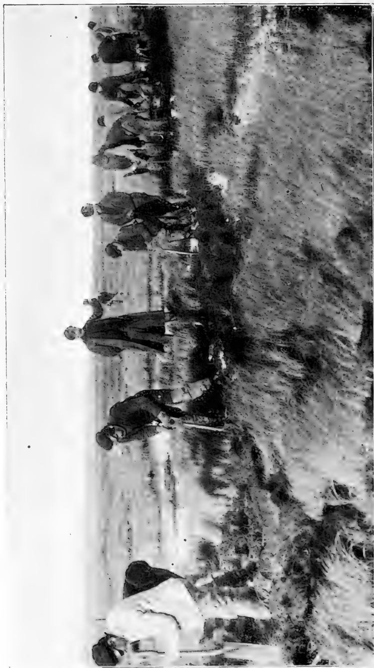
Fig. 4. A ditching gang at work on the Staten Island Marshes. From a photo made for Dr. A. H. Doty.
