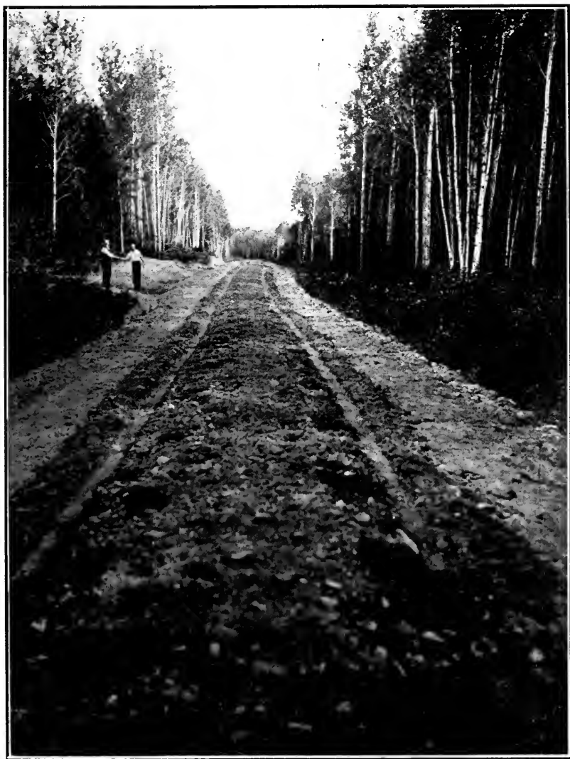
Gravelling a new road between Dryden and Wabigoon, in the District of Kenora.
