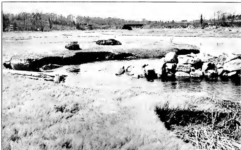
a. Broken dike, Stony Creek.
