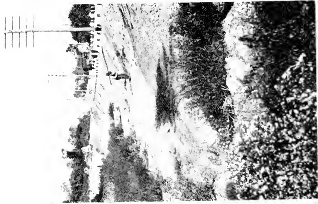
A TYPICAL VIEW OF THE FILL SLOPES ON THE PHILADELPHIA ROAD AFTER CONSTRUCTION
