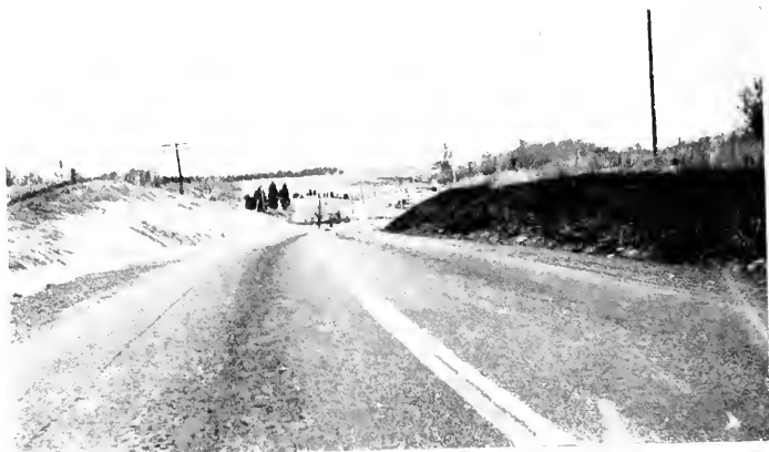
A SECTION WIDENED BY PRISON LABOR ON RT. 313 BETWEEN CHURCH HILL AND CHESTERTOWN IN QUEEN ANNE'S CO.
