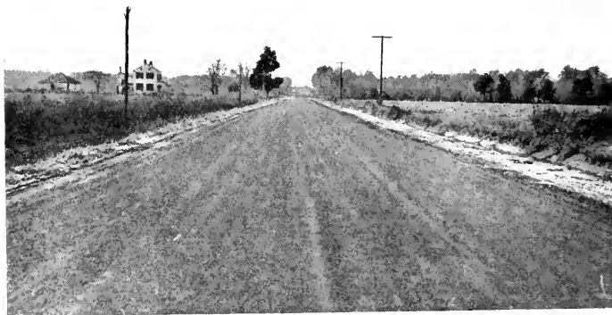
A BITUMINOUS-TREATED SECTION OF GRAVEL SURFACING ON A COUNTY HIGHWAY BETWEEN WHITE HAVEN AND CLARA IN WICOMICO COUNTY
