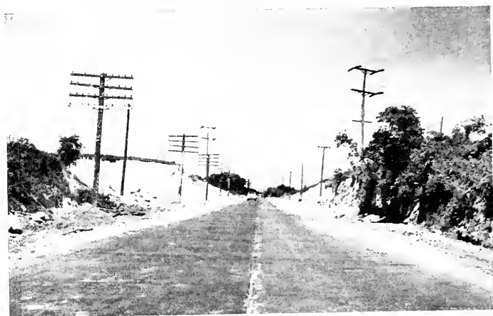
THE ELIMINATION OF THE "BOTTLENECK" BY A RELOCATION MADE BY THE FACILITIES OF THE WPA
