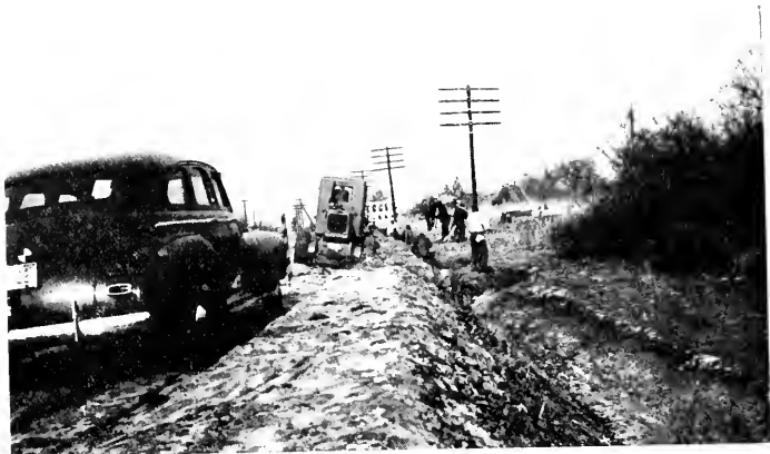
IMPROVING A DRAINAGE CONDITION BY PRISON LABOR BETWEEN DENTON AND GREENSBORO ON RT. 313 IN CAROLINE COUNTY
