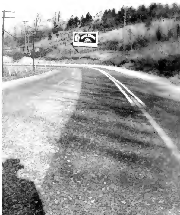
SHOWING WIDENED SECTION OF SURFACING ON THE WEST SLOPE OF BRADDOCK MT., ROUTE 40, IN FREDERICK COUNTY, TO CREATE A LANE FOR SLOW-MOVING VEHICLES
