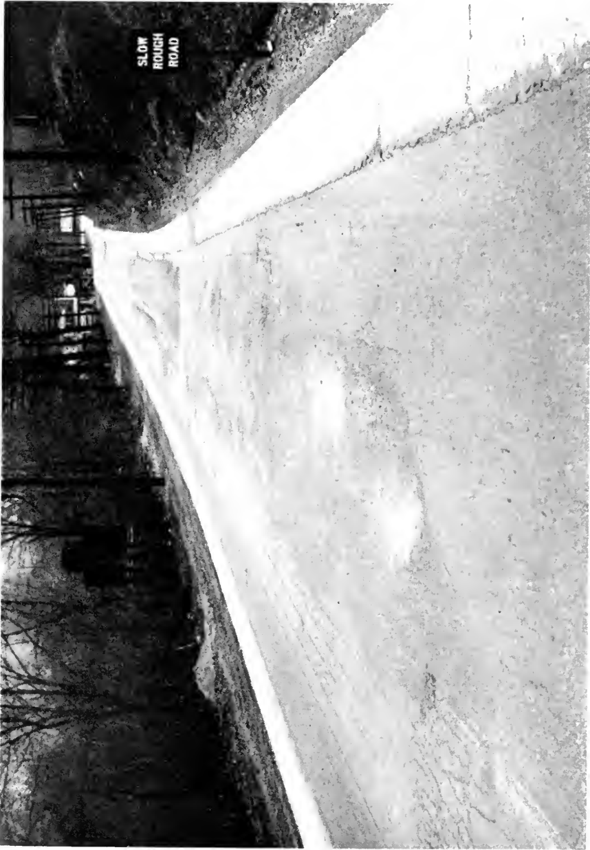
U. S. ROUTE 40 LOOKING EAST NEAR CLARYSVILLE SHOWING A SECTION OF BROKEN SURFACING CAUSED BY BASE FAILURES BECAUSE OF THE CONCENTRATION OF TRAFFIC IN THE WAR EFFORT
