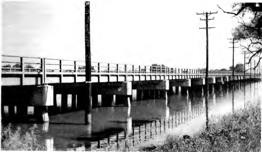
FOUR-LANE BRIDGE CARRYING EASTERN AVENUE OVER BACK RIVER, NEAR ESSEX, IN BALTIMORE COUNTY
