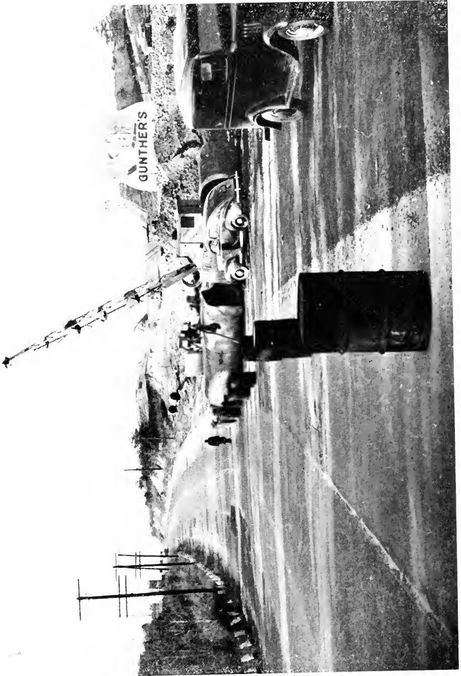
THE CONSTRUCTION OF THE RELOCATION WHICH WILL ELIMINATE DEAD MAN'S CURVE ON THE BALTIMORE-WASHINGTON BOULEVARD
