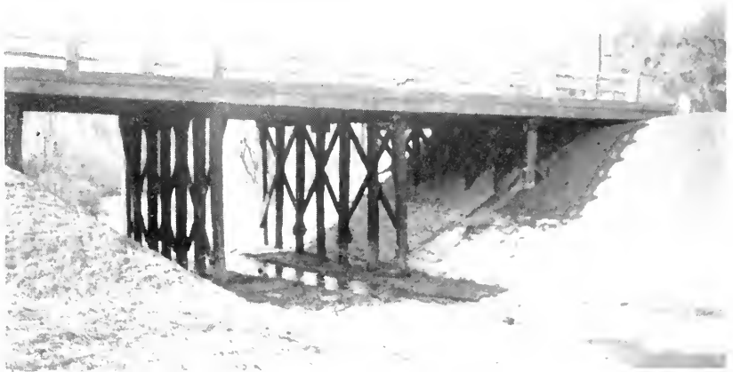
A TREATED TIMBER BRIDGE OVER COSTER'S CREEK ON ROUTE 2 IN CALVERT COUNTY
