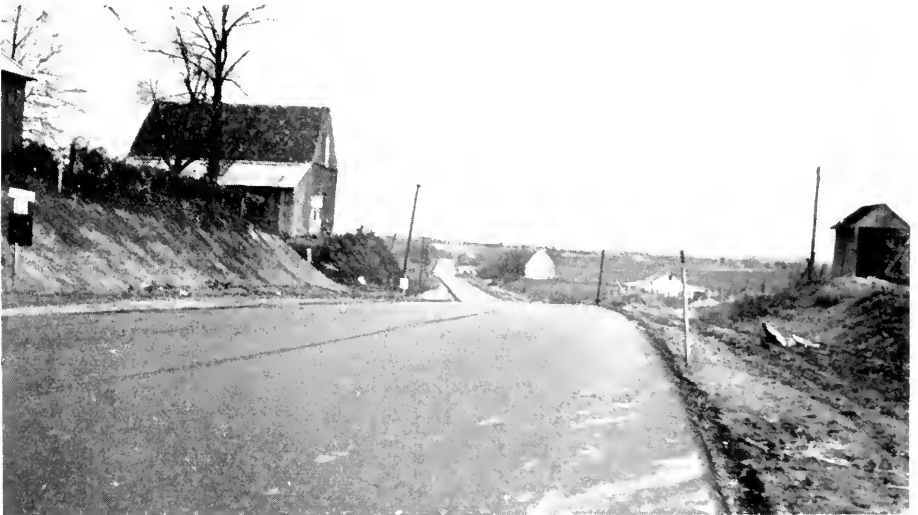
A VIEW ON THE DAVIDSONVILLE ROAD AT THE SAME POINT AFTER RESURFACING AND WIDENING FROM 16 FEET TO 24 FEET AND DURING THE CONSTRUCTION OF THE 12-FOOT SHOULDERS
