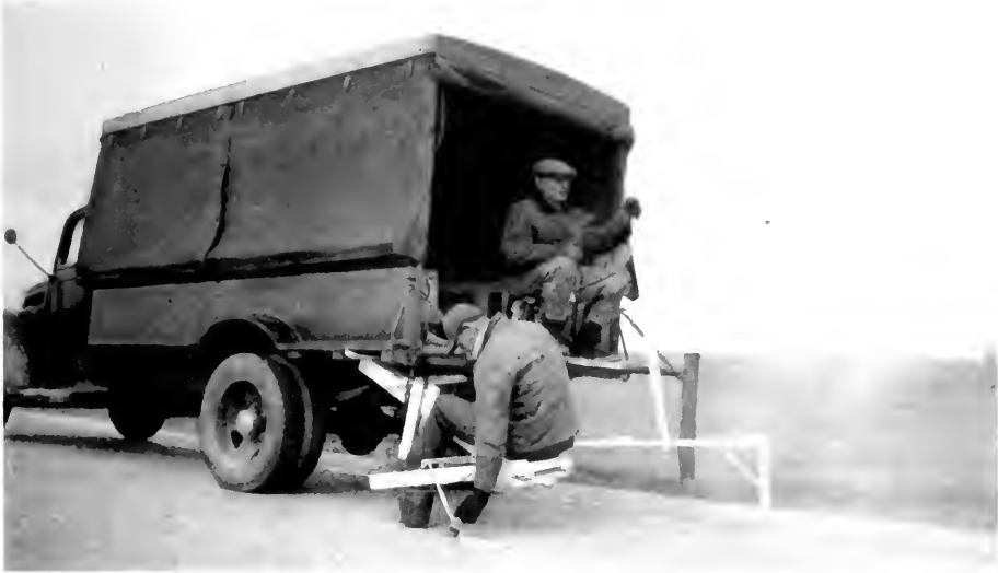
IMPROVISED METHOD FOR SPOTTING ROADS TO BE CENTER-LINE STRIPED IN DISTRICT No. 2
