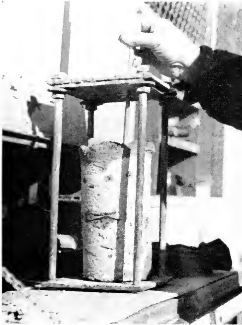
THE THICKNESS OF PAVING IS DETERMINED FROM THE EXTRACTED CORE: TEN MEASUREMENTS MADE AT MATHEMATICALLY DERIVED LOCATIONS ARE AVERAGED FROM EACH CORE—CORE DRILL TRUCK
