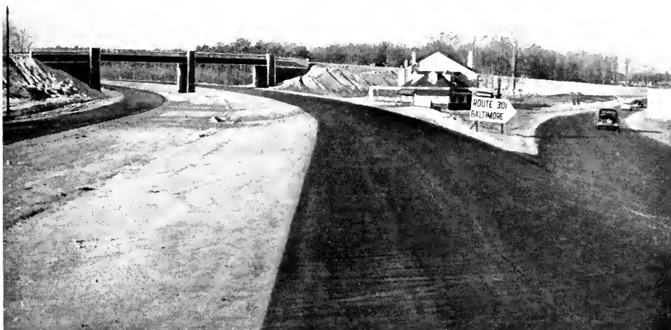
AFTER IMPROVEMENT—INTERCHANGE AREA AT U. S. ROUTE 301 AND MD. ROUTE 5 AT T.B. MARYLAND
